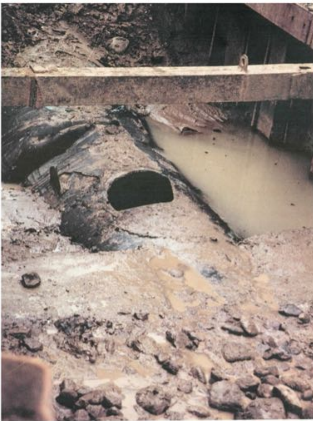
Damaged pipe section - broken out to allow for emptying
