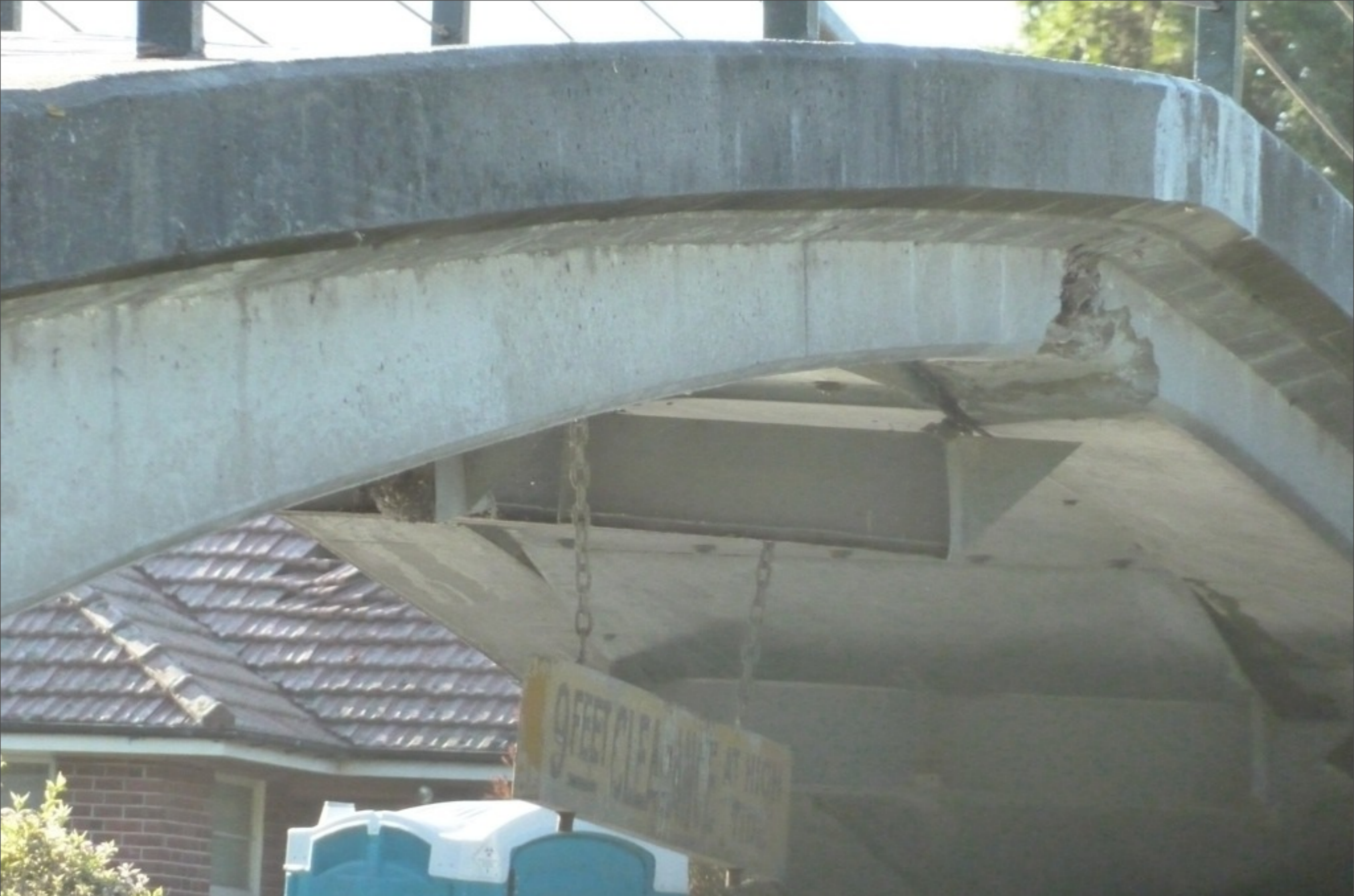
2011: More lateral Spreading, now forming a 3-pin arch
