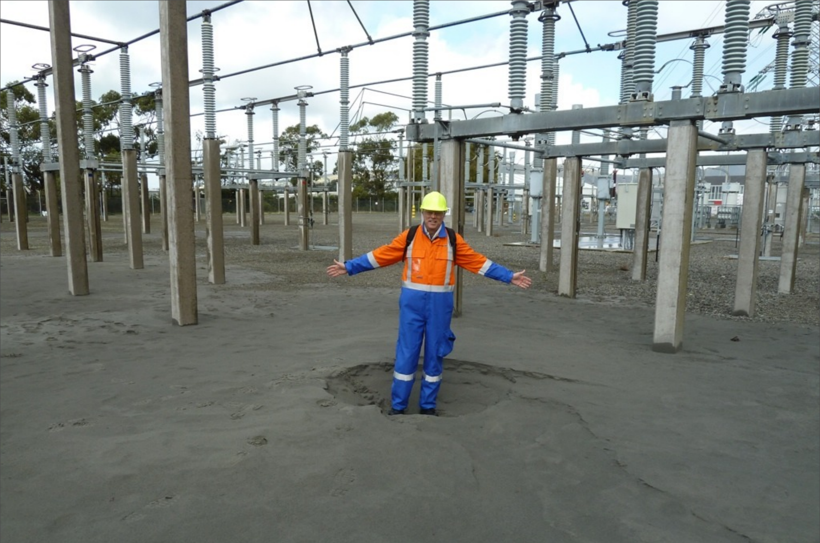
Large sand boil in 220 kV Yard
