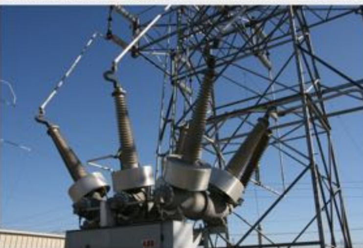
bushwork failed in 2007 EQ
