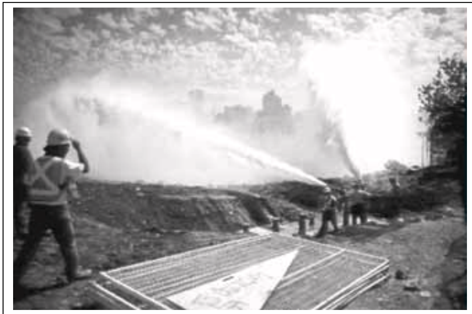
Figure 12-5 Vancouver, B.C. DFPS (a) False Creek pump station (foreground, nearing completion in 1995); (b) welded steel pipe under construction, 1995; (c) False Creek station proof test, 1995.
