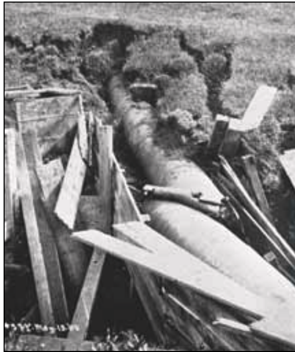
Figure 2-8 Failure of Pilarcitos 30 inch pipeline. Pipe telescoped and was thrown sideways on the wooden bridge crossing Small Frawley Canyon. San Andreas fault crosses pipe diagonally.
