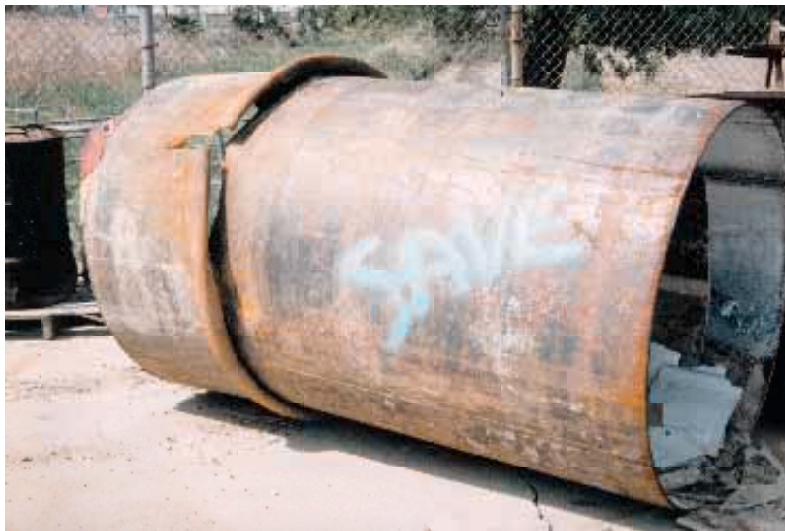
Figure 6-3. Wrinkled 48" Balboa Boulevard Pipeline. This pipe leaked
