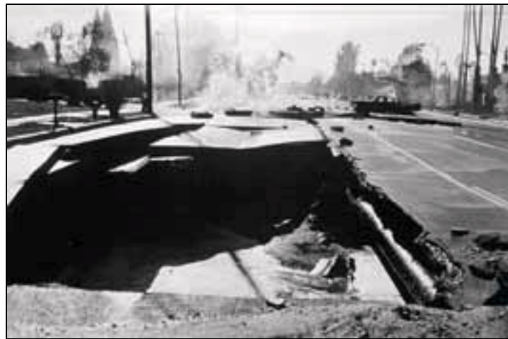
Figure 2-21 North Balboa Blvd. Incident, 1994 Northridge Earthquake (top) Aerial View, (bottom) Surface View
