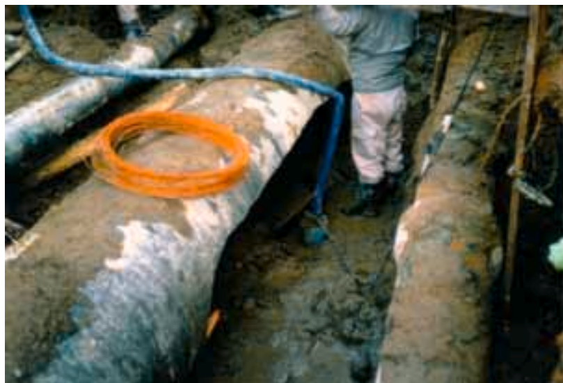
Figure 6-6. Damaged Pipeline, Kobe 1995
