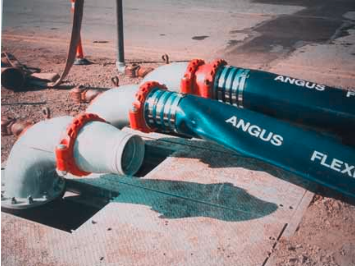
Figure 13-2. Flex Hose Deployment in EBMUD System
