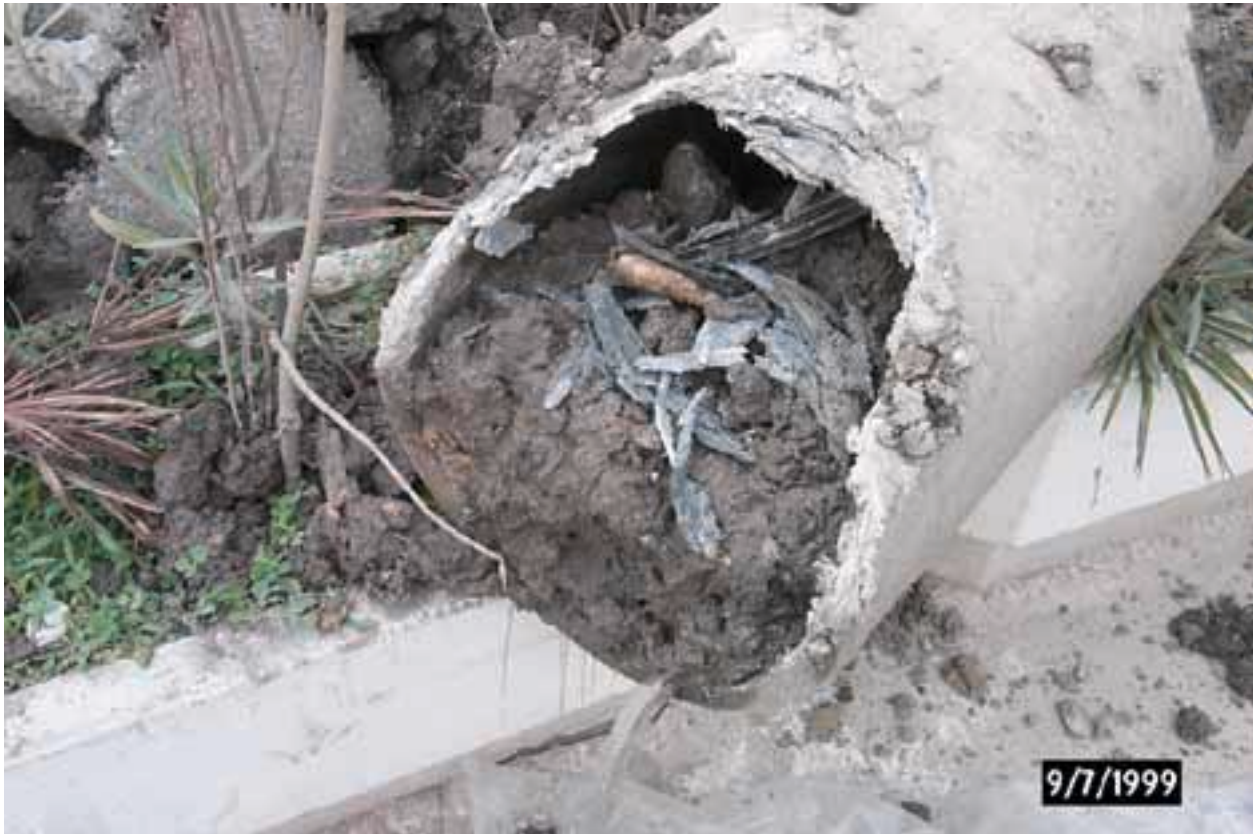
Figure 6-7. Damaged AC Pipeline, Adapazari, Turkey 1999
