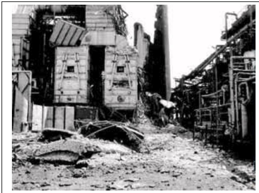
Figure 2-24 Tupras Refinery damage due to fire following earthquake (a) Burnt and collapsed tank; (b) Top of stack collapsed into unit, severely damaging heater unit. Top of stack is in foreground of photo.
