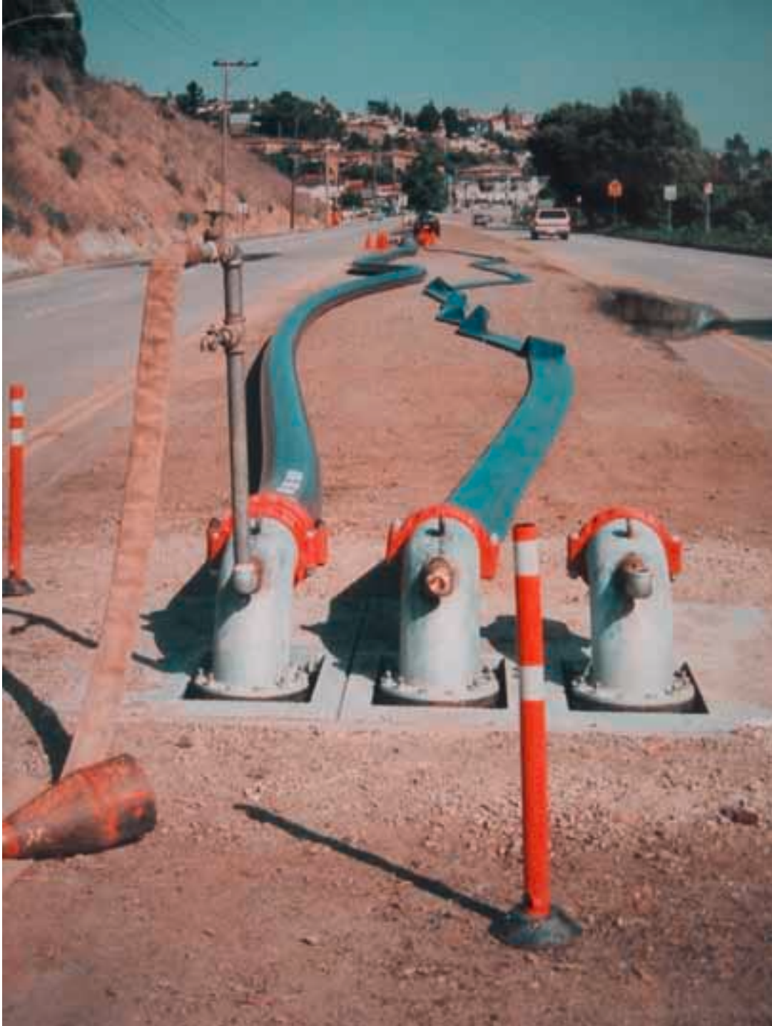
Figure 13-1. Flex Hose Deployment in EBMUD System
