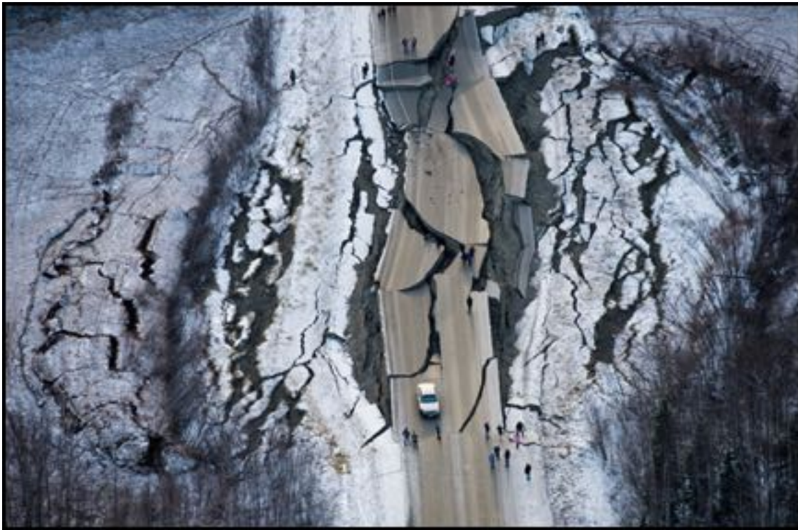
Figure 6.36-2. Roadway Deformations (December 1 2018)
