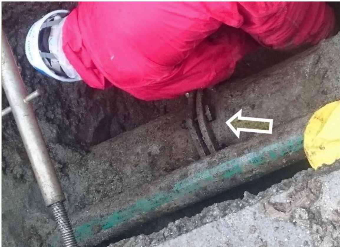
Figure 6.34-1. Repair to medium pressure steel pipe; repair was to tighten the mechanical joint (typical of 9 locations)
