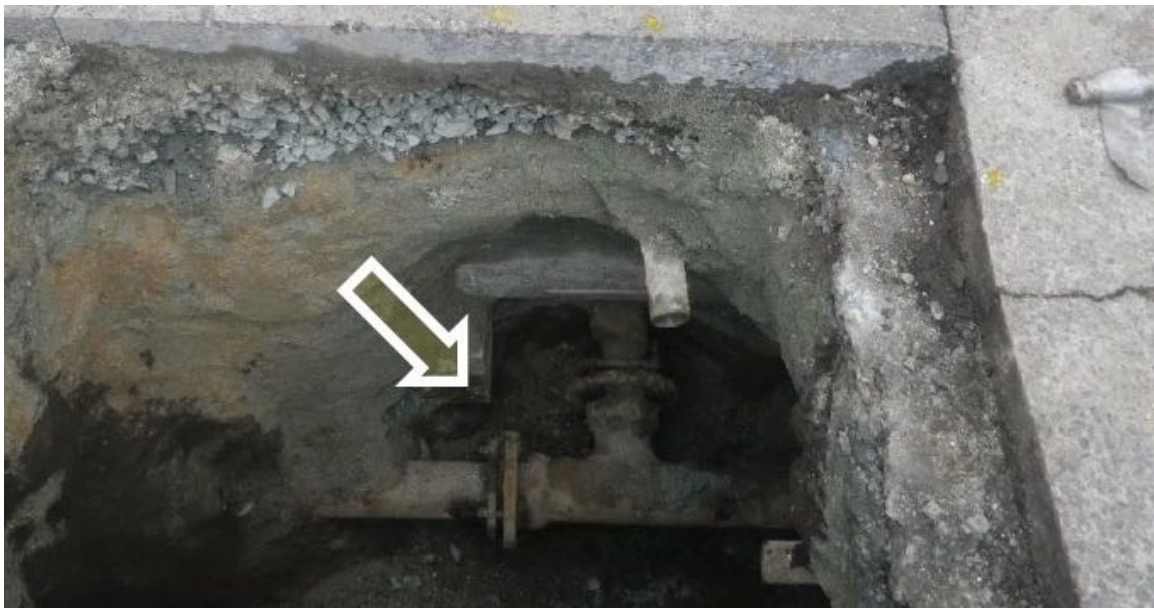
Figure 6.34-2. Repair to low pressure distribution steel pipe; repair was to tighten the mechanical joint (typical of 23 locations)
