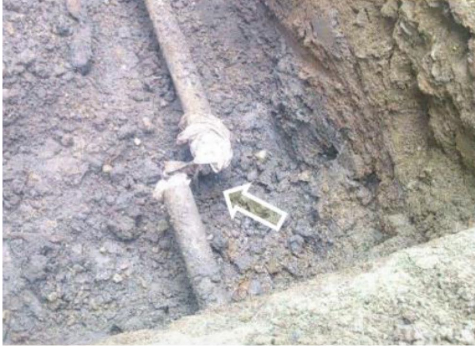
Figure 6.34-3. Repair to low pressure distribution steel screwed joint pipe; repair was to tighten the mechanical joint
