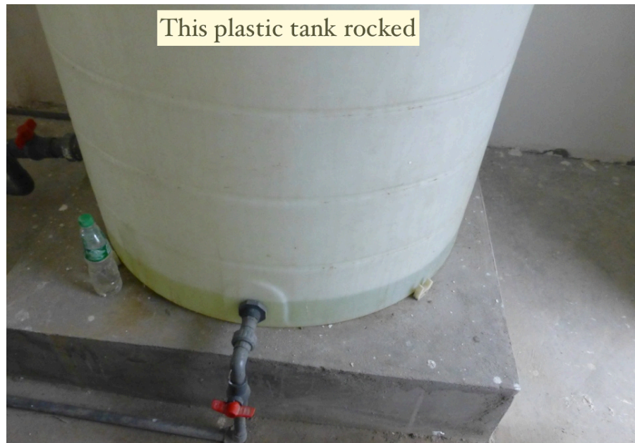
Figure 10. Plastic Tank for Chlorine Dioxide Disinfectant
