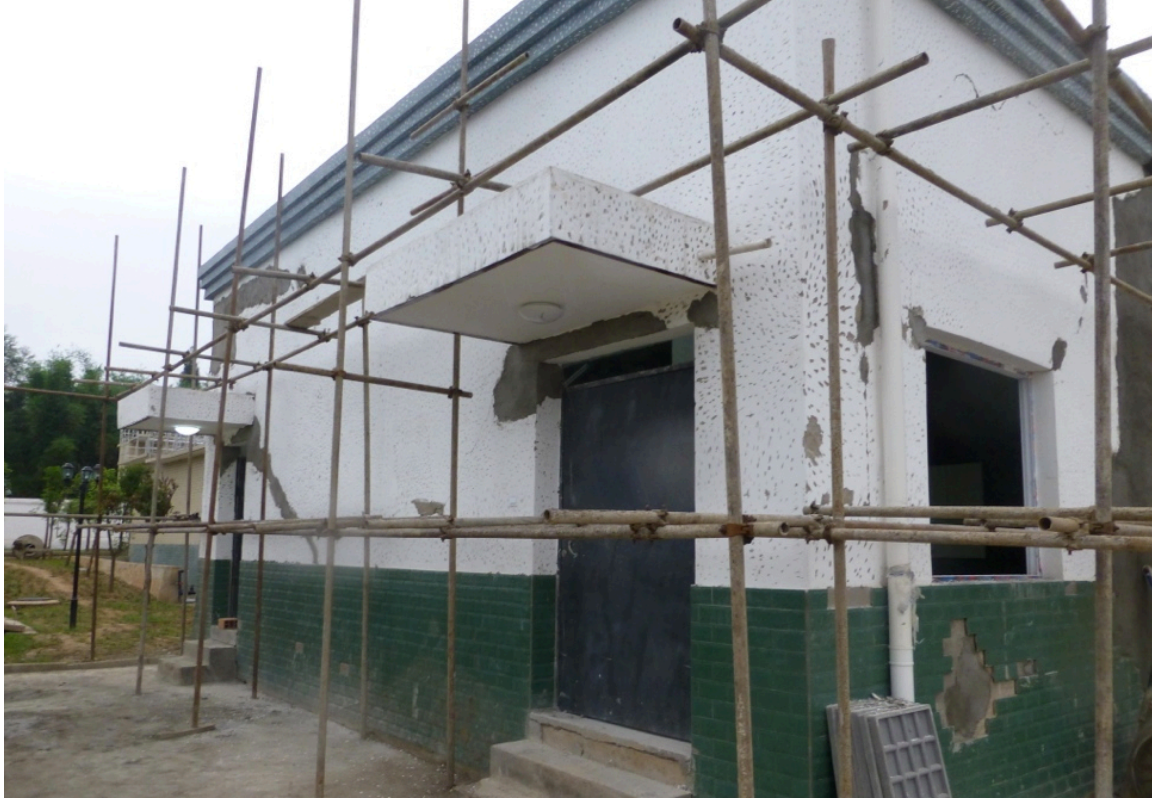
Figure 9. Damaged Control Building
