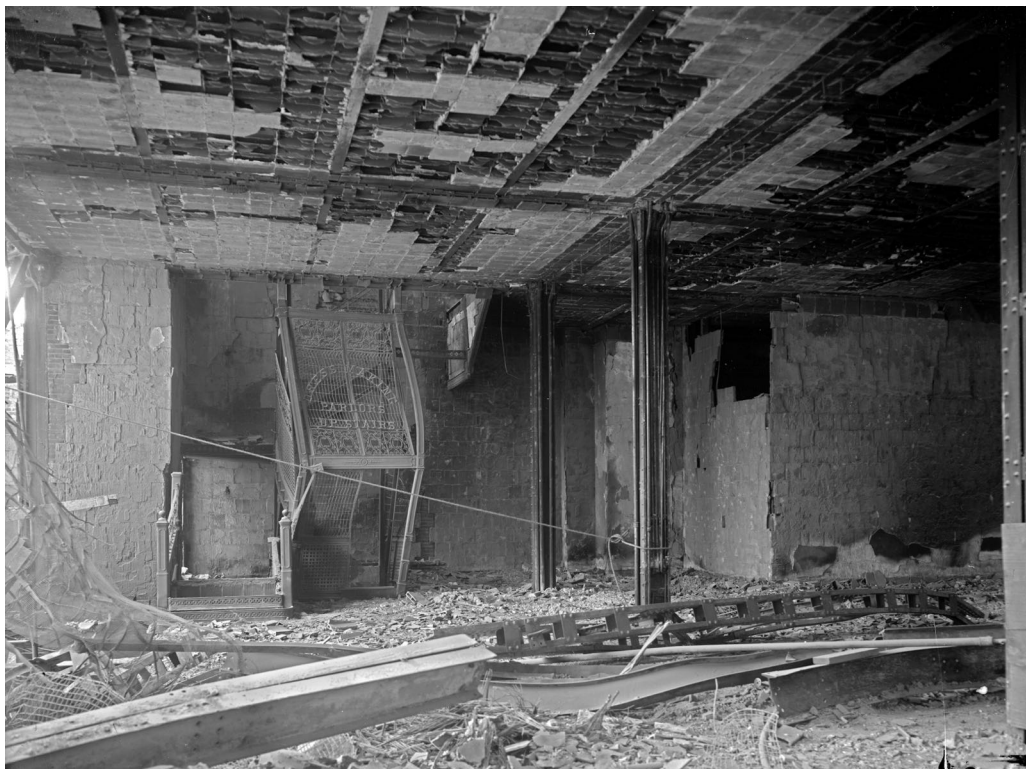
Figure 4.7-3. Interior of SVWC Office Building after 1906 earthquake (photo: Courtesy Mike Housh, SF Historian)
