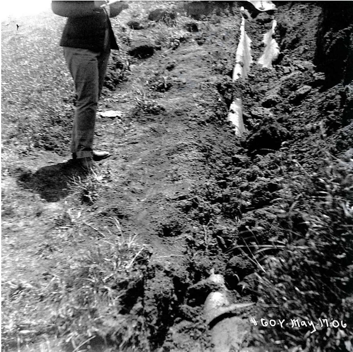
Figure 4.1.3-2. Failure of Pilarcitos 30 inch pipeline about 220 yards south of FX-1. Pipe is collapsed on itself. Looking southerly. (Photo: Schussler 1906)
