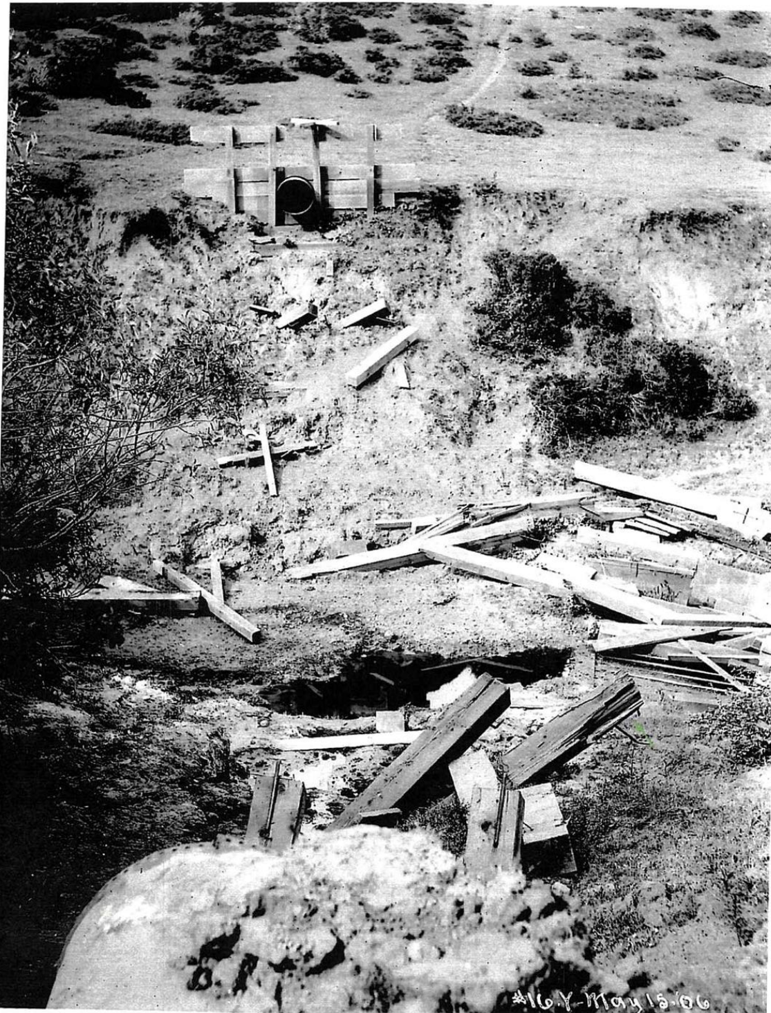
Figure 4.1.1-1. Large Frawley Canyon. Destruction of heavy bridge and 30-inch Pilarcitos pipe over Large Frawley Canyon. The pipe was torn in three locations and thrown sideways over 50 feet to the east into the canyon below. View looking northerly. (Photo: Schussler 1906, HS8)
