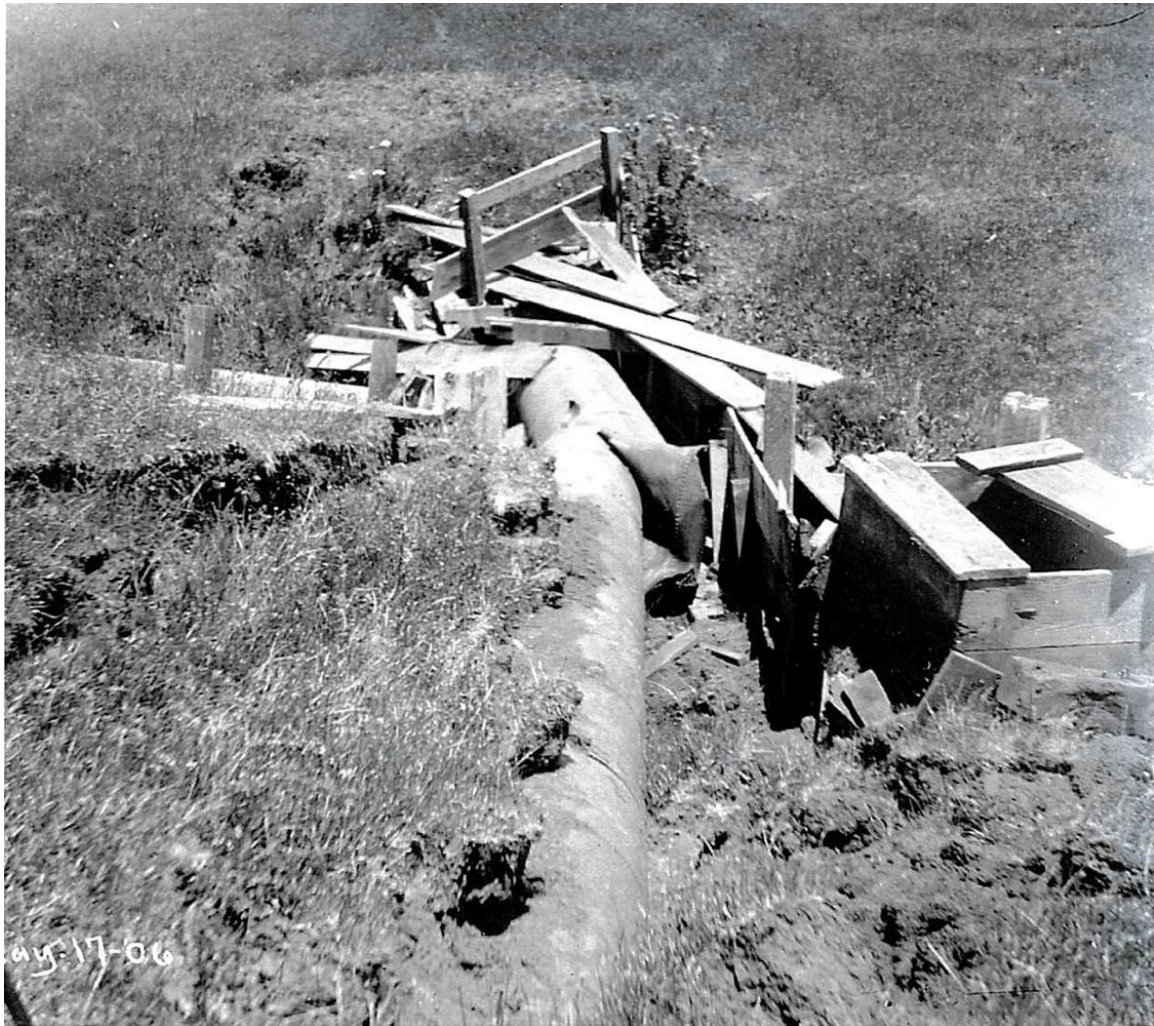
Figure 4.1.2-3. Failure of Pilarcitos 30 inch pipe. Pipe telescoped and was thrown sideways off the wooden bridge crossing Small Frawley Canyon. View looking north. (Photo: Schussler 1906)
