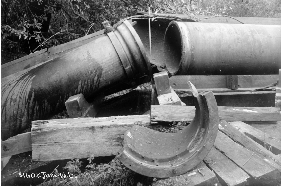
Figure 4.1.14-3. Crossing 5. 24" Pilarcitos Cast Iron Pipe. Elbow crushed. View looking north. (Photo: Schussler 1906 HS11)
