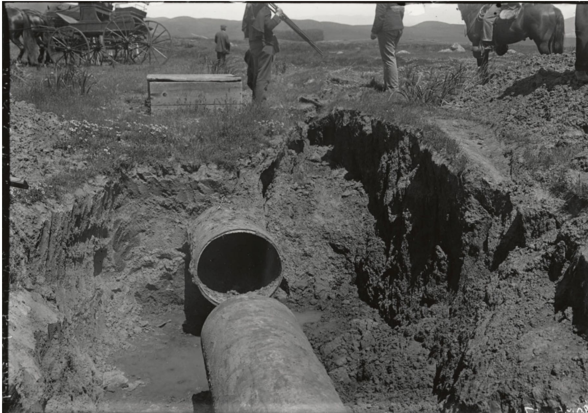
Figure 4.1.8-3. FX-4. Failure of Pilarcitos 30 inch pipeline. At north end of San Andreas Reservoir (Photo: Lawson 1908)
