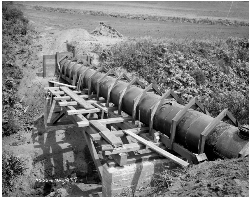
Figure 4-4. Construction of the Baden-Merced 30-inch Pipe at Creek Crossing (using former Pilarcitos Pipe segments) (1907)
