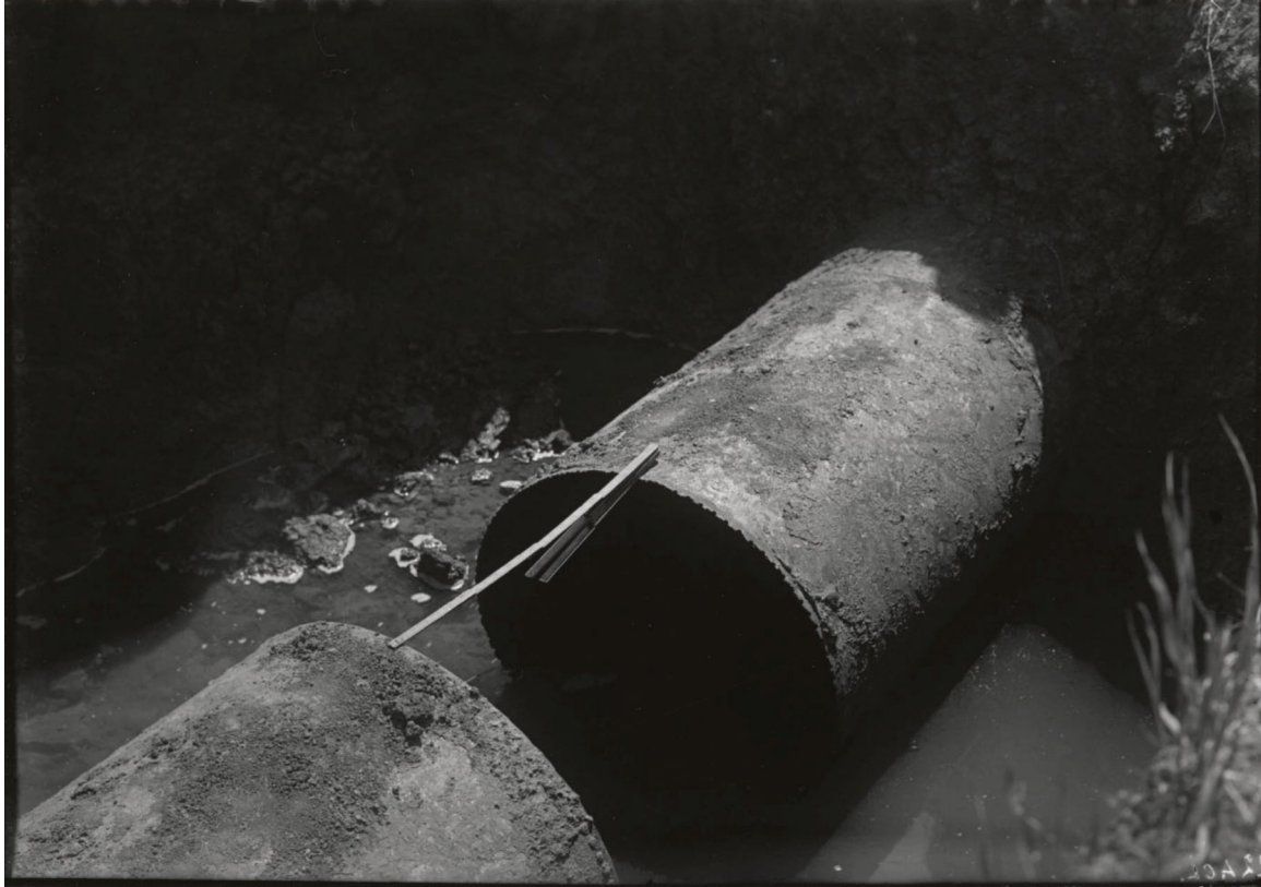
Figure 4.1.8-6. Failure of Pilarcitos 30 inch pipe at FX-4. Pull Apart ~ 21.5 inches. Note edge distance tears at rivets. (Photo credit: Lawson, 1908)
