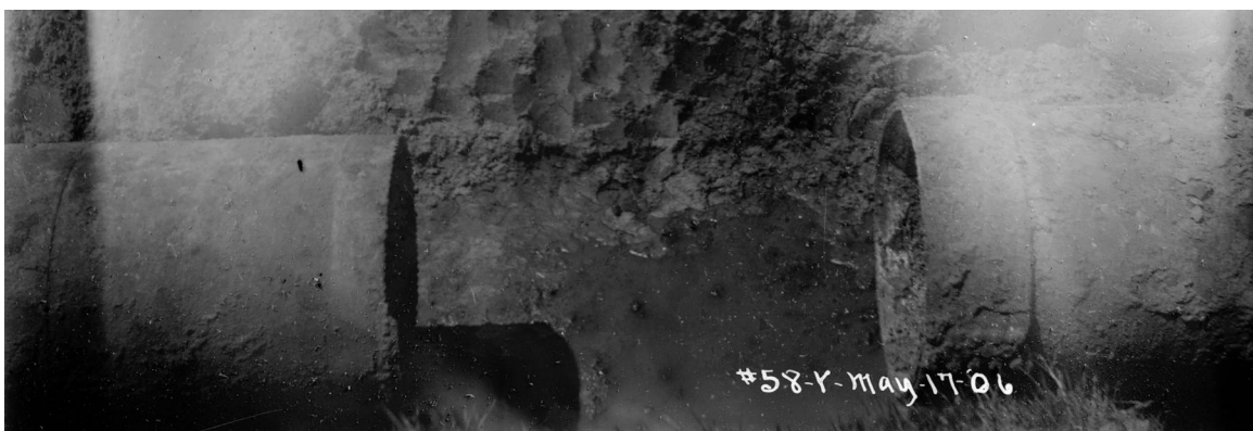
Figure 4.1.8-4. Crossing 4. Failure of Pilarcitos 30 inch pipeline. Looking Westerly (Photo: SVWC 1906)
