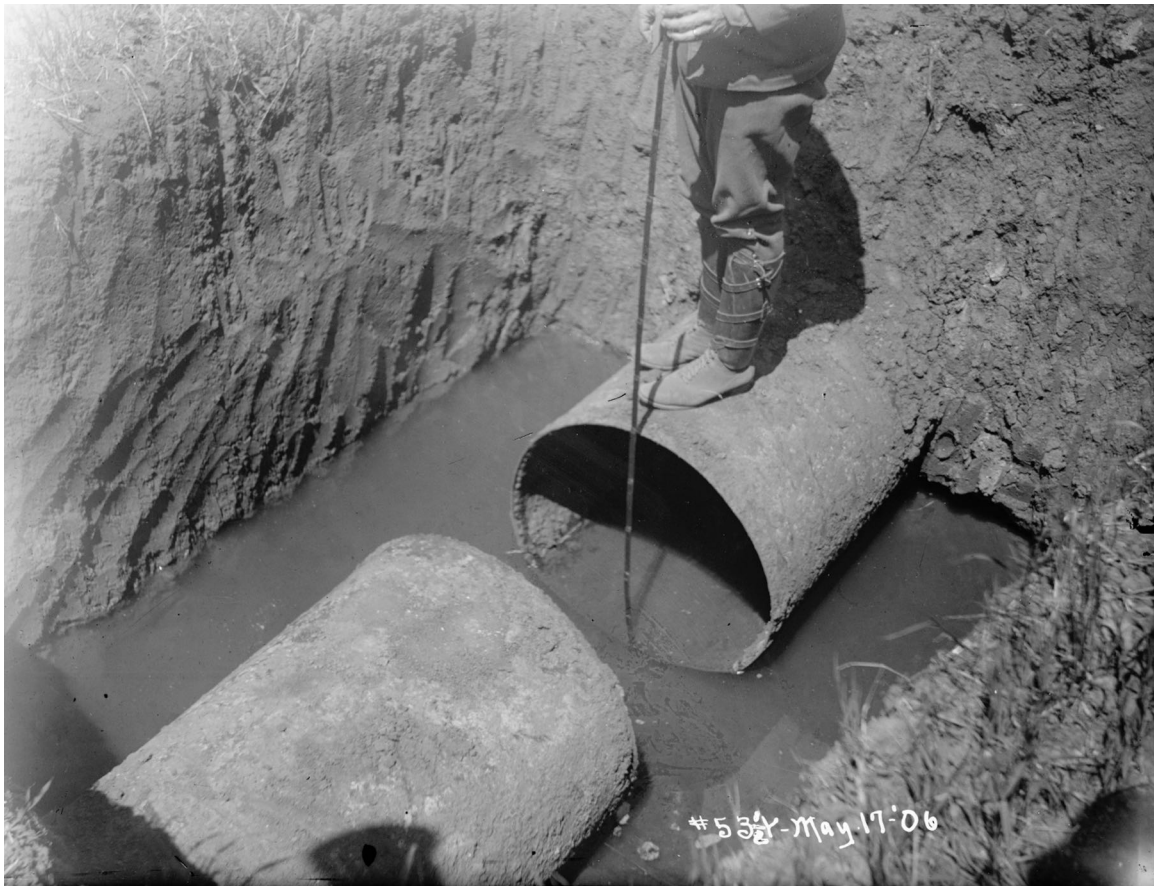
Figure 4.1.8-5. Site 8. Failure of Pilarcitos 30 inch pipeline. Pull Apart ~ 21.5 inches. (Photo Credit Schussler HS3 1906)
