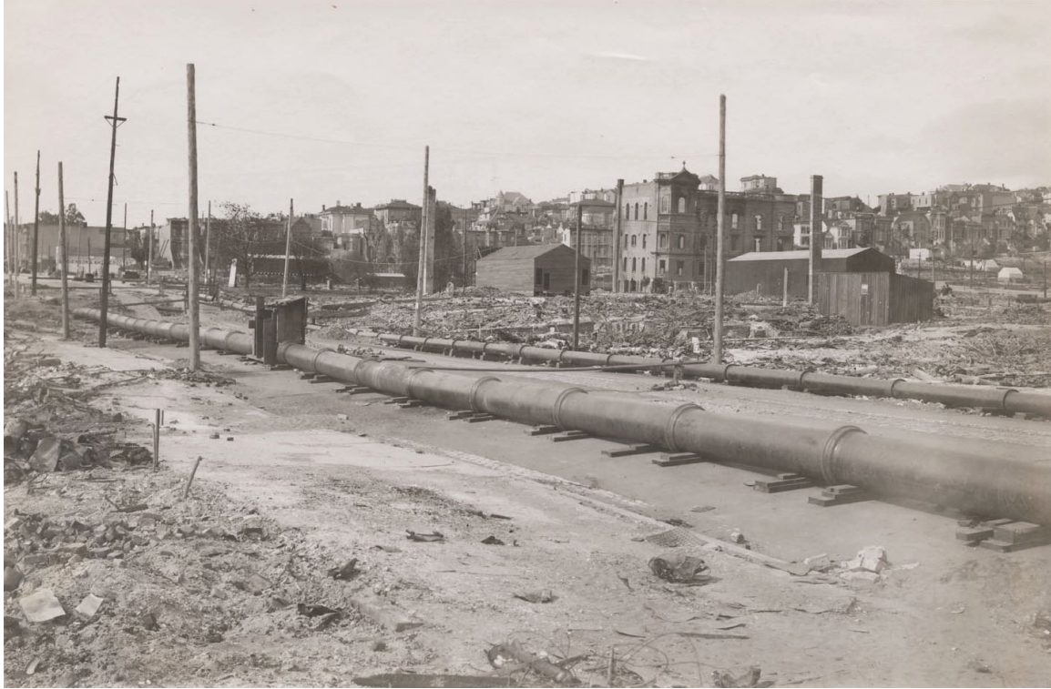
Figure 7-49. c. May 16 1906. View of Valencia Street between 18 th and 19 th street, looking southwesterly. The two temporary pipes are cast iron with belled joints; no restraints are seen placed across the segmented joints. Each segment is typically supported by two sets of wooden planks. (Photo credit: Online Archive of California, The 1906 San Francisco Earthquake and Fire Digital Collection, U. C. Berkeley, Bancroft Library)
