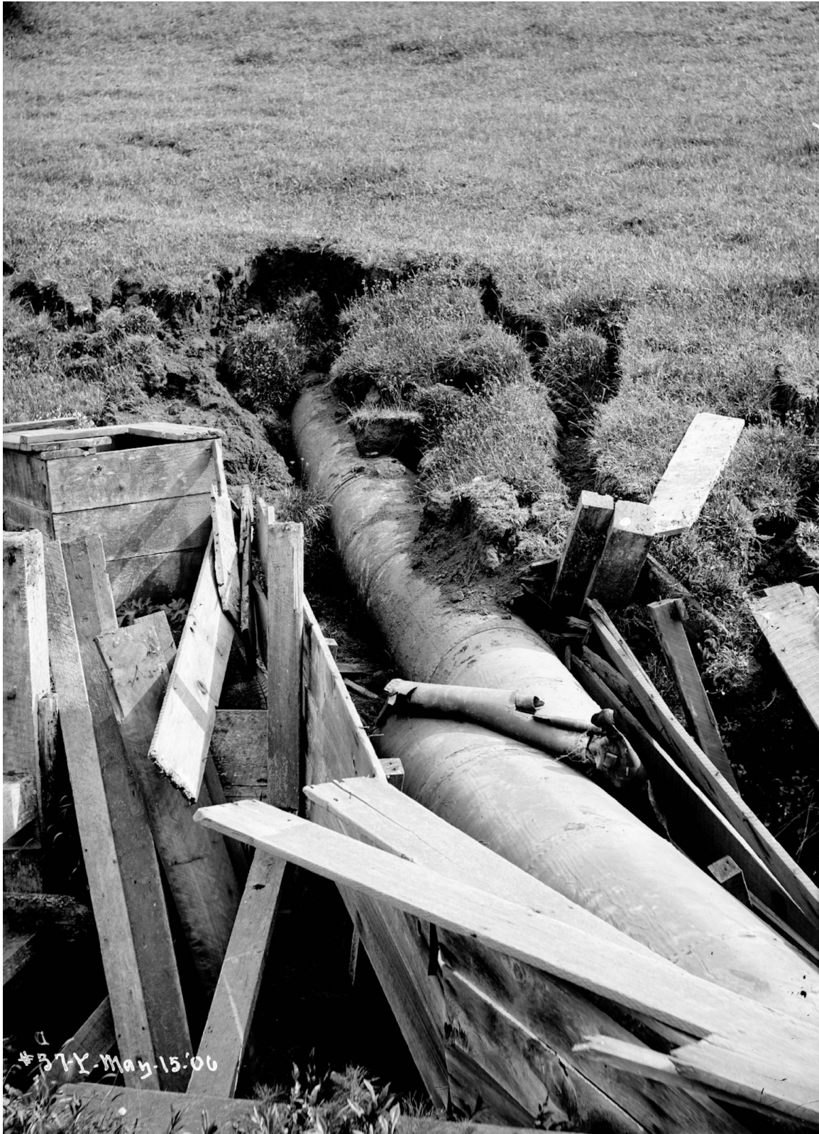
Figure 4.1.2-1. Small Frawley Canyon. Failure of Pilarcitos 30 inch pipe. Pipe is telescoped and thrown sideways on bridge over Small Frawley Canyon. View looking south. (Photo: Schussler 1906, HS5)
