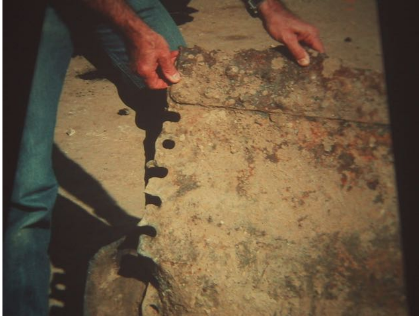
Figure 6-2. Close Up View of Damaged LADWP Riveted Pipe, 1994
