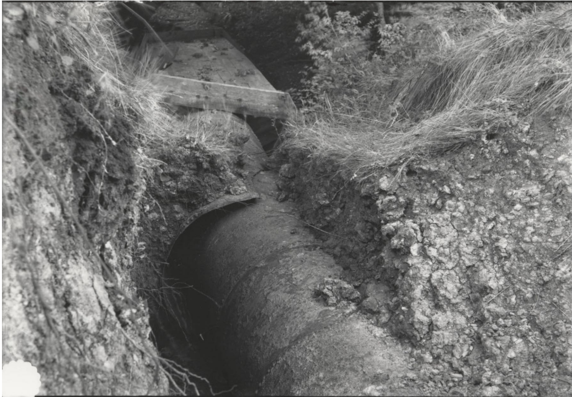
Figure 4.1.18-4. Wrought Iron Pipe Failure. Site 18 (Photo: SVWC, 1906?)
