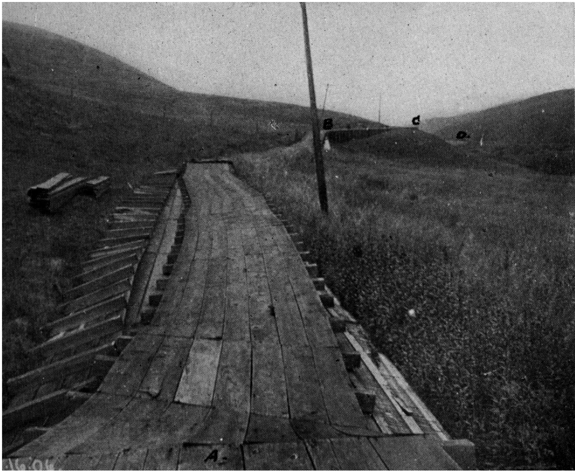
Figure 4.1.12-10. Failure of Stone Dam Flume, Looking Southerly (Photo: Schussler 1906 HS49)
