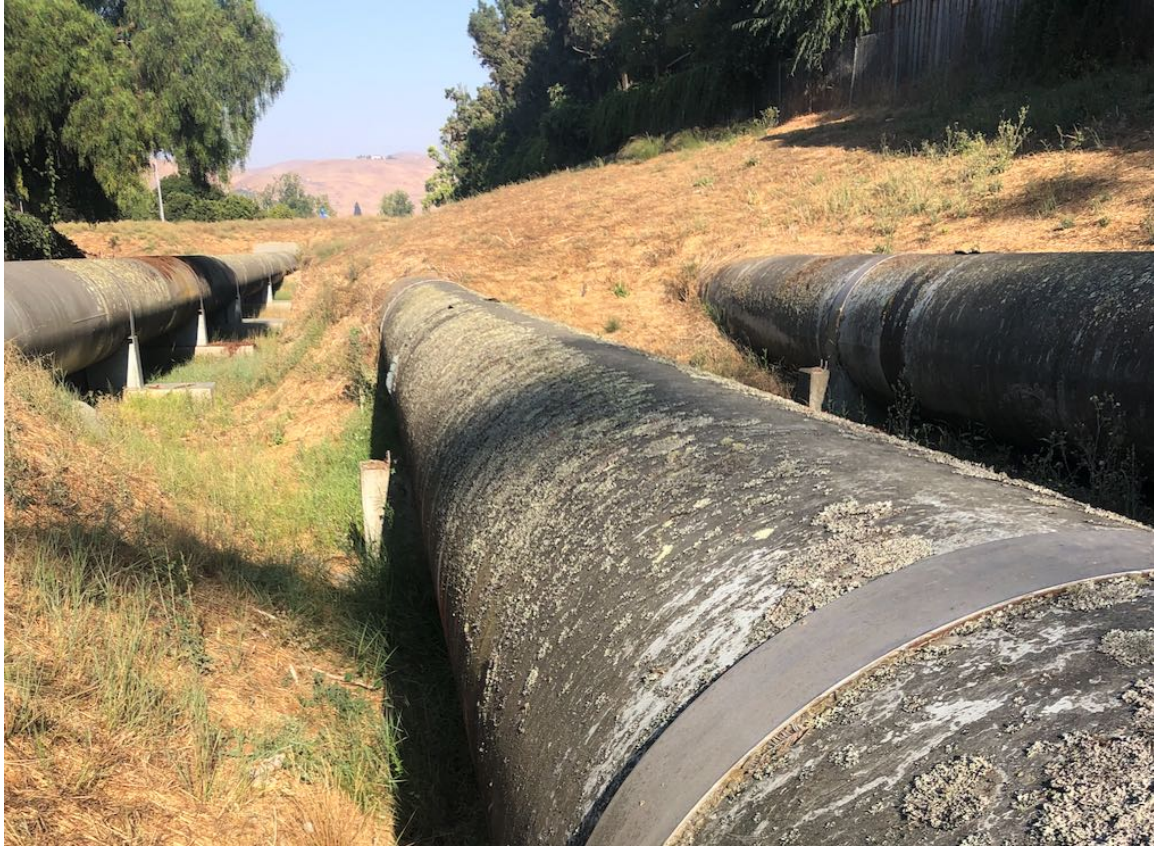
Figure 6-4. SFPUC's Hetch Hetchy Aqueduct BDPL 1, 2, 5 Pipelines where they cross the Hayward fault in Frmont (2023)
