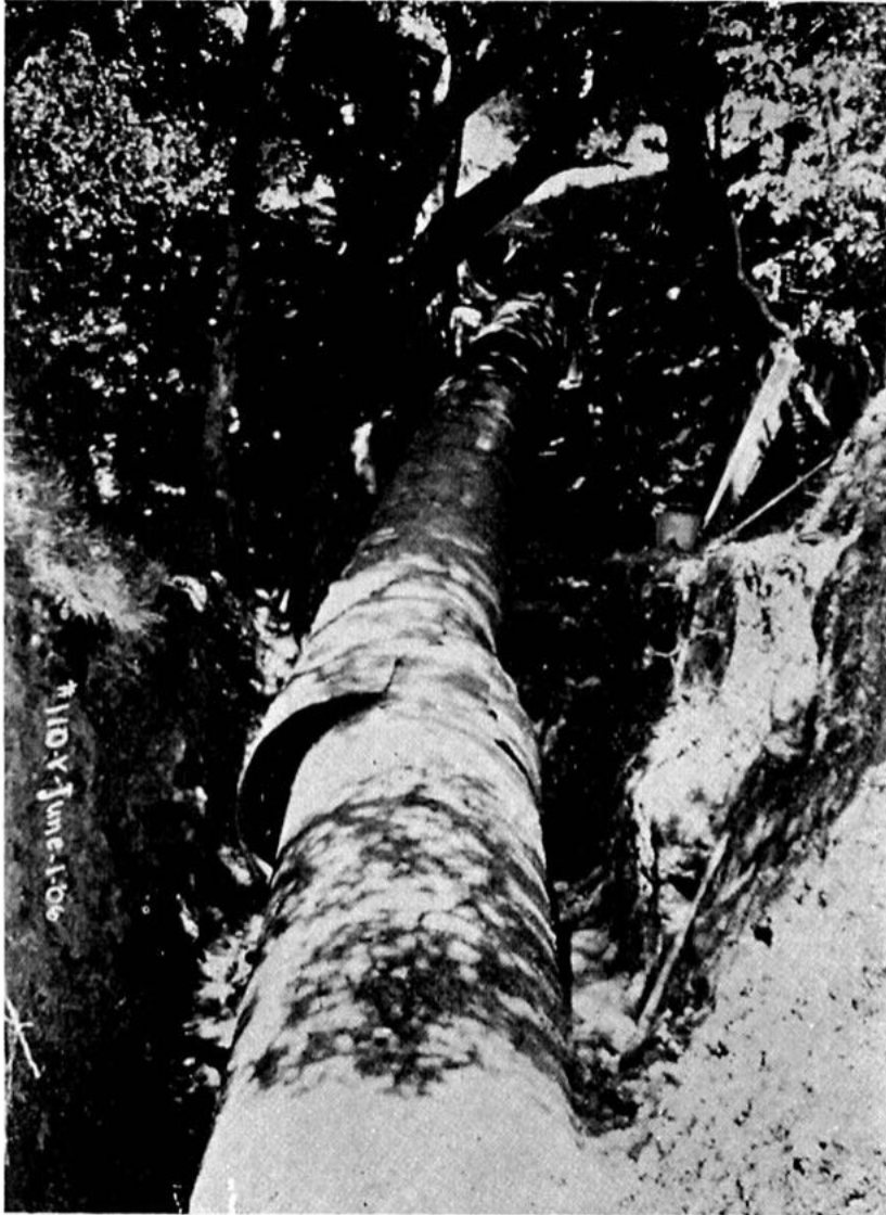
Figure 4.1.17-3. FX-6. Locks Creek 44" Wrought Iron Pipe is offset to the north about 14" and telescoped about 51". Looking easterly. Location is about 50 feet east of the County road between the San Andreas and Crystal Springs reservoirs. (Photo: Schussler 1906 HS14)
