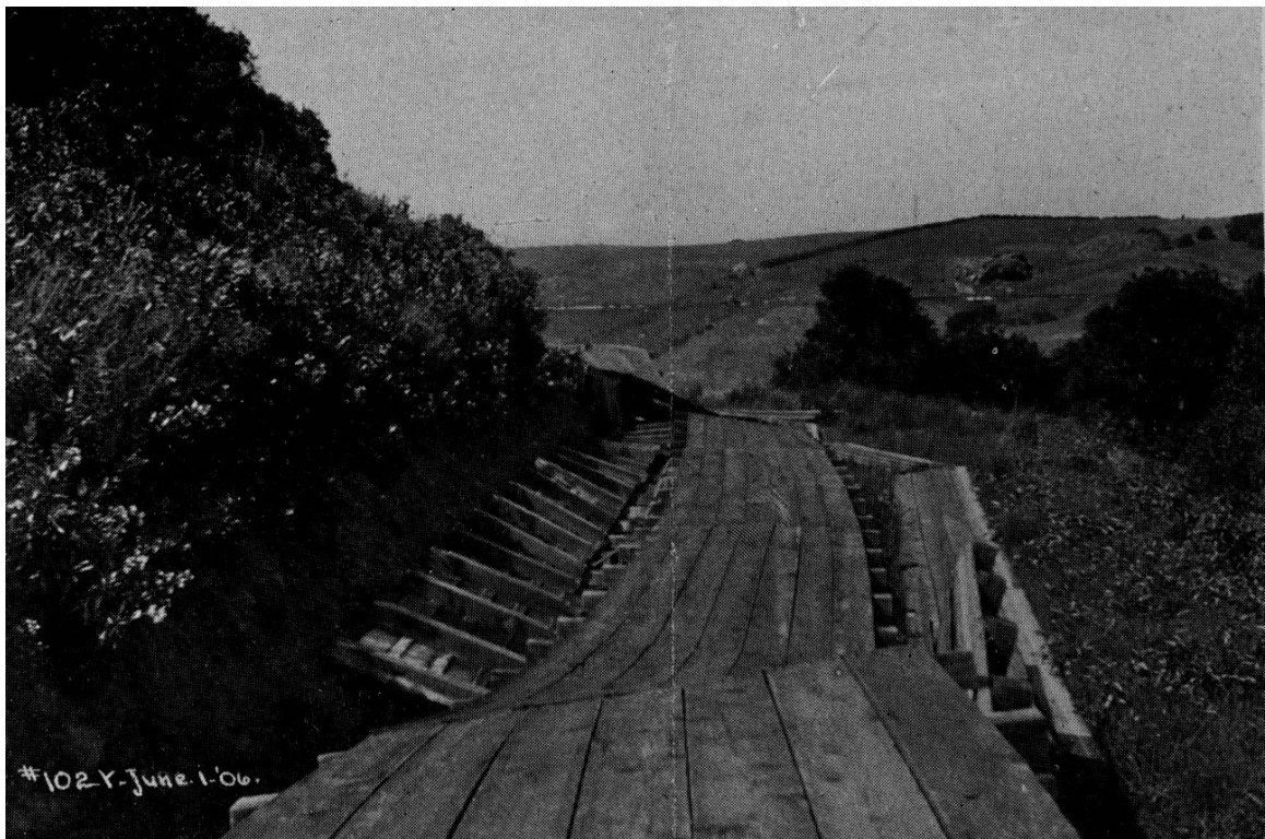
Figure 4.6-3. Failure of Pilarcitos Waste Water Flume to San Andreas Reservoir, Looking Northerly (Photo: Schussler 1906 HS47)
