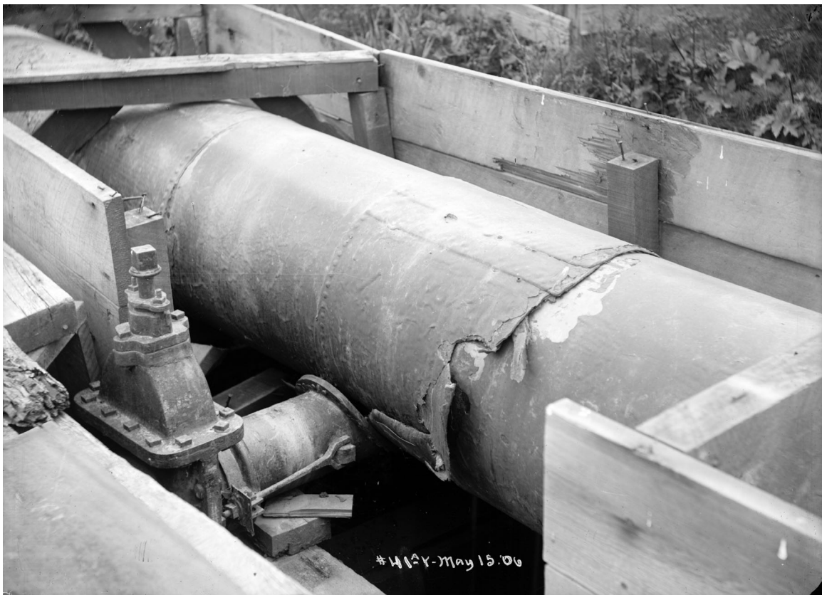
Figure 4.1.7-1. South of FX-3. Pipe has telescoped 58" on the trestle. Just south of Sneath Rancho. Looking northerly. (Photo: Schussler 1906 HS1)
