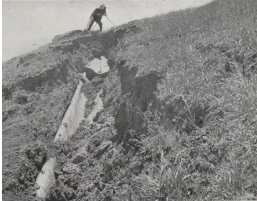
Figure 4.1.3-3. Vacuum Failure of Pilarcitos 30 inch pipeline; same location as 4.1.3-1. South of the failure at FX-1, Small Frawley Canyon (Photo RLH)
