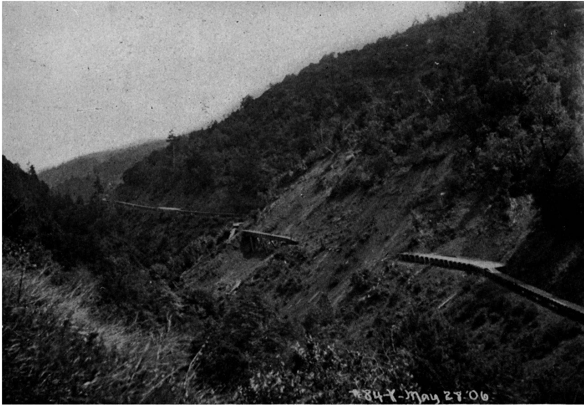
Figure 4.6-5. Collapse of Pilarcitos Side Flume between (here 5' x 3') in Upper San Mateo Canyon. Photo dated May 27 1906. (Photo: SVWC).
