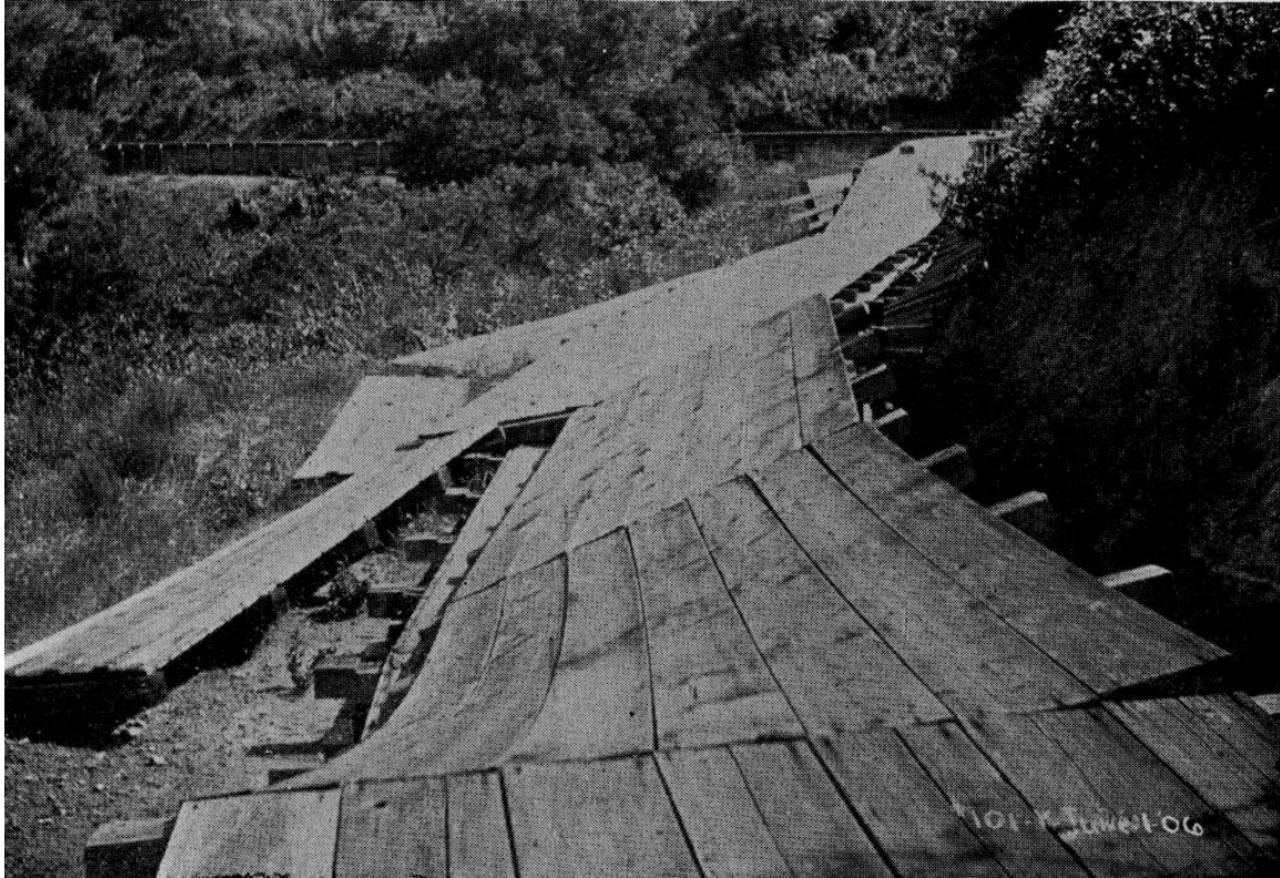
Figure 4.6-4. Failure of Pilarcitos Waste Water (Side) Flume to San Andreas Reservoir, Looking Southerly (Photo: Schussler 1906 HS48)
