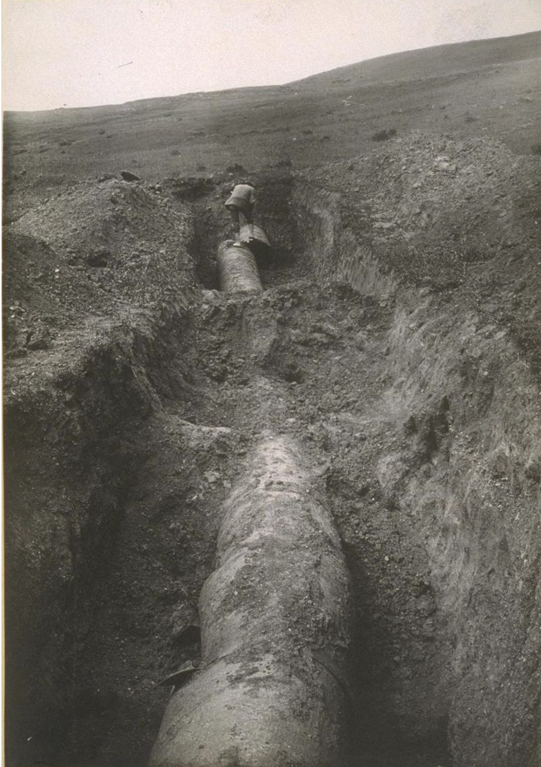
Figure 4.1.6-1. FX-3. View North. South end telescoped 21". The north end moved 17" west and telescoped 41". (Photo: Derleth 1907. See Also Schussler 1906 HS2 for similar photo)
