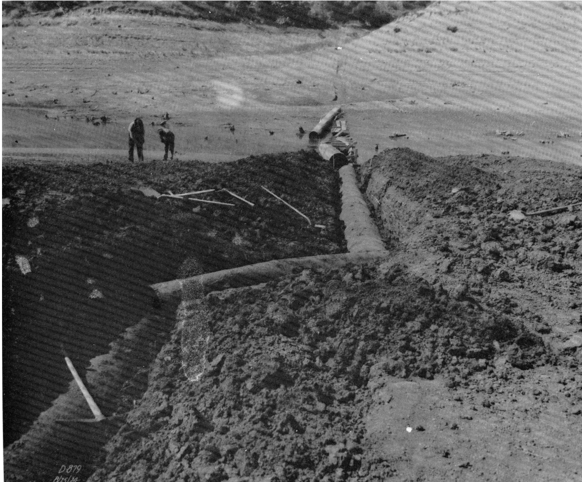
Figure 4.1.18-2. 37" Abandoned Pipe, 8-25-1924, D-879 (Credit: SVWC 1924). Looking West
