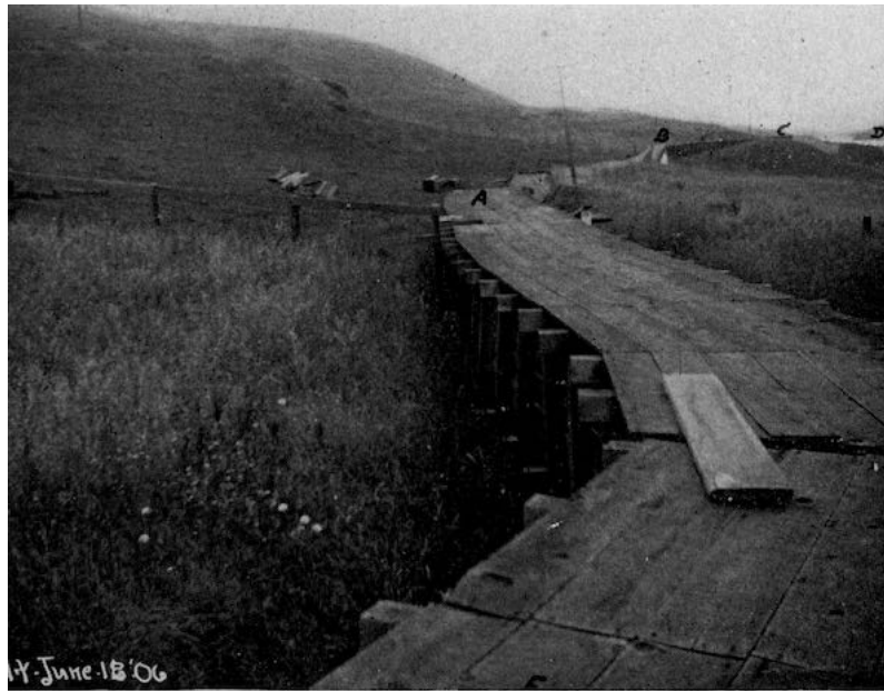
Figure 4.1.12-9. Failure of Stone Dam Flume, Looking Southerly (Photo: Schussler 1906 HS50)
