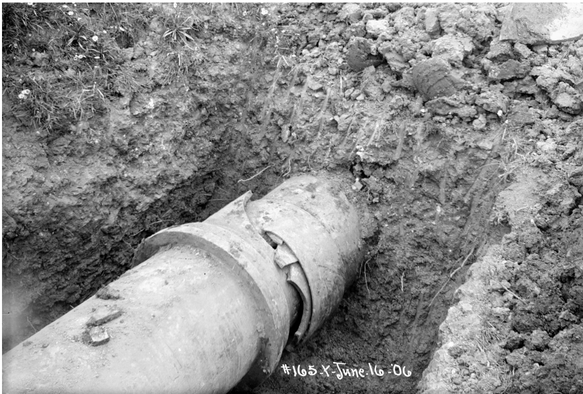
Figure 4.1.14-5. FX-5. 24" Pipe has telescoped \pm 1' . About 100' north of FX-5. (Credit: Schussler 1906 HS13)
