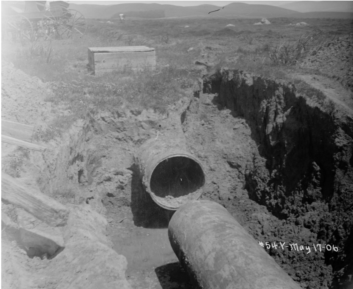
Figure 4.1.8-1. FX-4. Failure of Pilarcitos 30 inch pipeline. At north end of San Andreas Reservoir. Looking Northwesterly. Pull Apart ~59". North segment of pipe is ~4" to the right (transverse) of the south segment. (Photo: Schussler HS7 1906)
