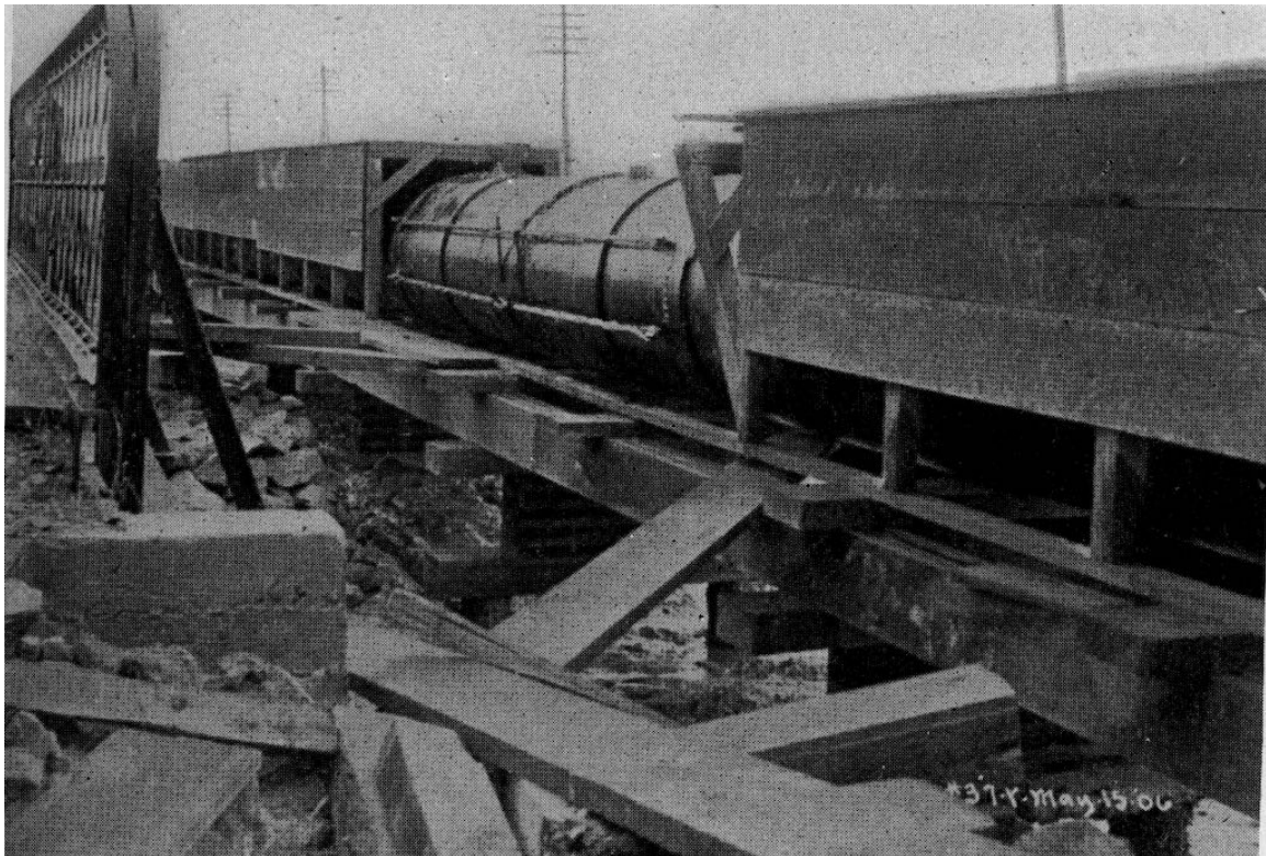
Figure 4.3-13. Crystal Springs 44" at San Bruno Marsh, showing original pile foundation and caps. The plank stringers and blocking are made of 2x12 redwood, spiked cross and lengthwise and 6x12 pine caps. (Trestle 12) (Photo: Schussler 1906 HS23)
