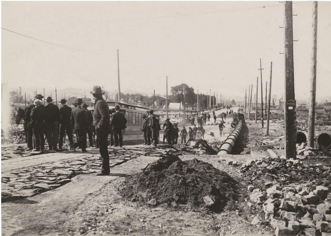
Figure 7-48. c. May 16 1906. View of Valencia Street between 18 th and 19 th street, looking south. In the center is an above-ground pipe laid by SVWC as a temporary bypass of the broken buried pipes. Several extra segments of temporary pipe are seen; pipe joints are apparently unrestrained, not an ideal situation for an above ground pipe, but theoretically feasible over a short straight run. (Photo credit: Online Archive of California, The 1906 San Francisco Earthquake and Fire Digital Collection, U. C. Berkeley, Bancroft Library)
