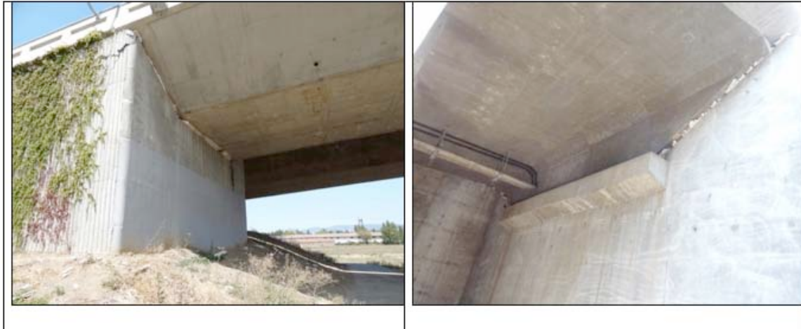
Figure 5-16. Outside and Inside of an abutment on the Napa River (West Imola Avenue) Bridges
