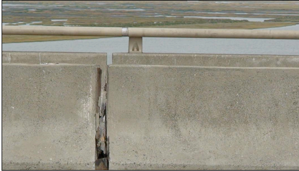
Figure 5-10. Damage to the Napa River Bridge was Permanent Longitudinal Displacement at the Expansion Joints
