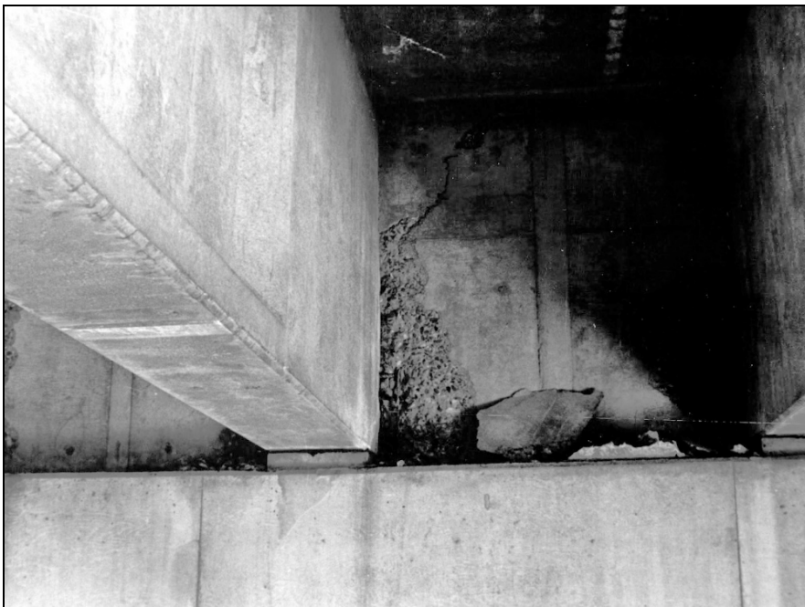
Figure 5-5. Damage to Napa River Bridge during the Loma Prieta 1989 Earthquake
