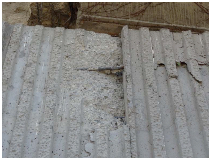
Figure 5-17. Close-up of damaged curtain walls on the Napa River (West Imola Ave) Bridge
