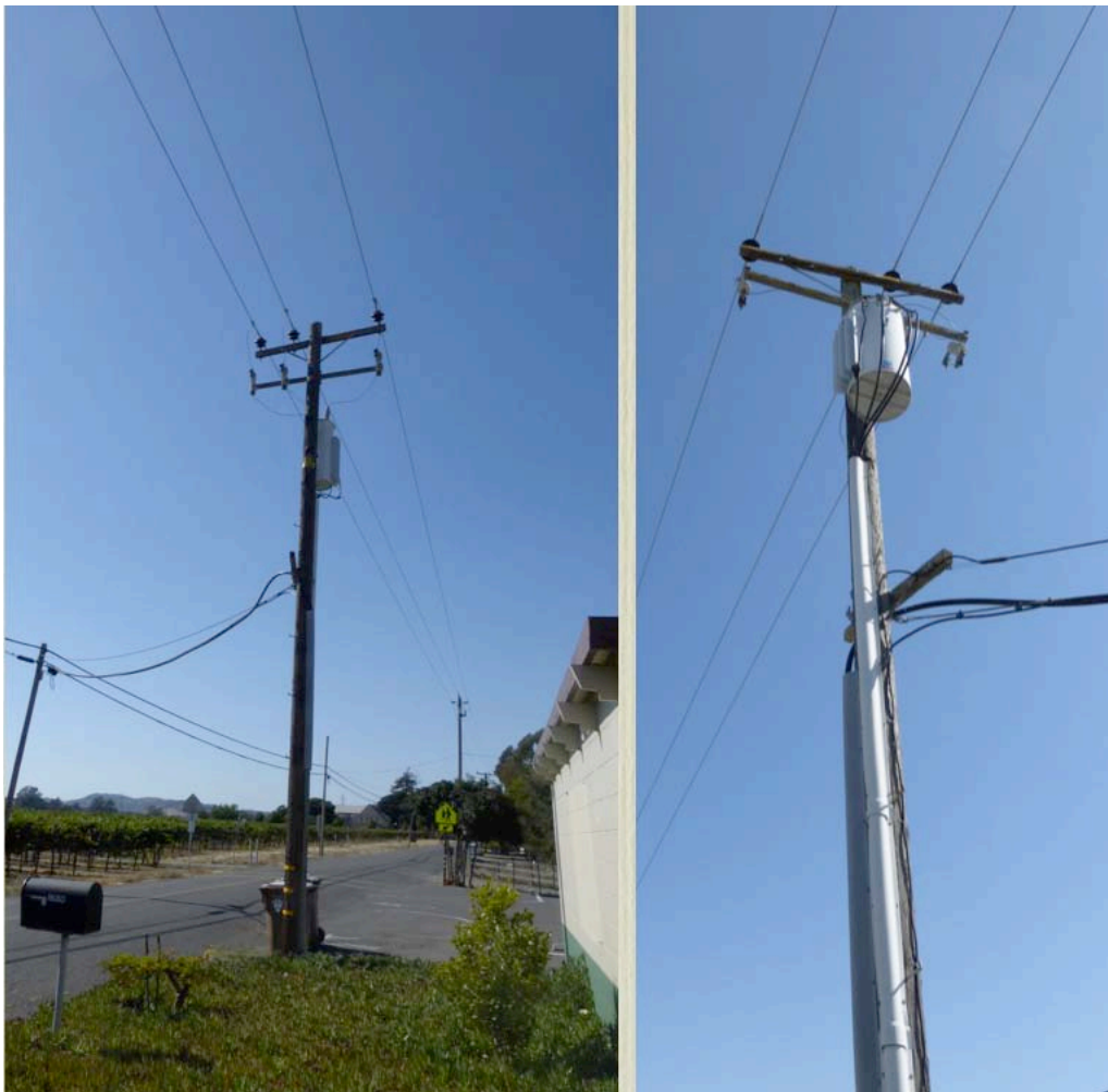
Figure 2-29. Power Pole, adjacent to fault zone (left side looking north, right side looking south)
