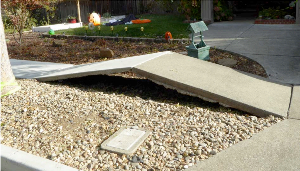
Figure 2-20. Buckled Sidewalk at Fault Offset Location
