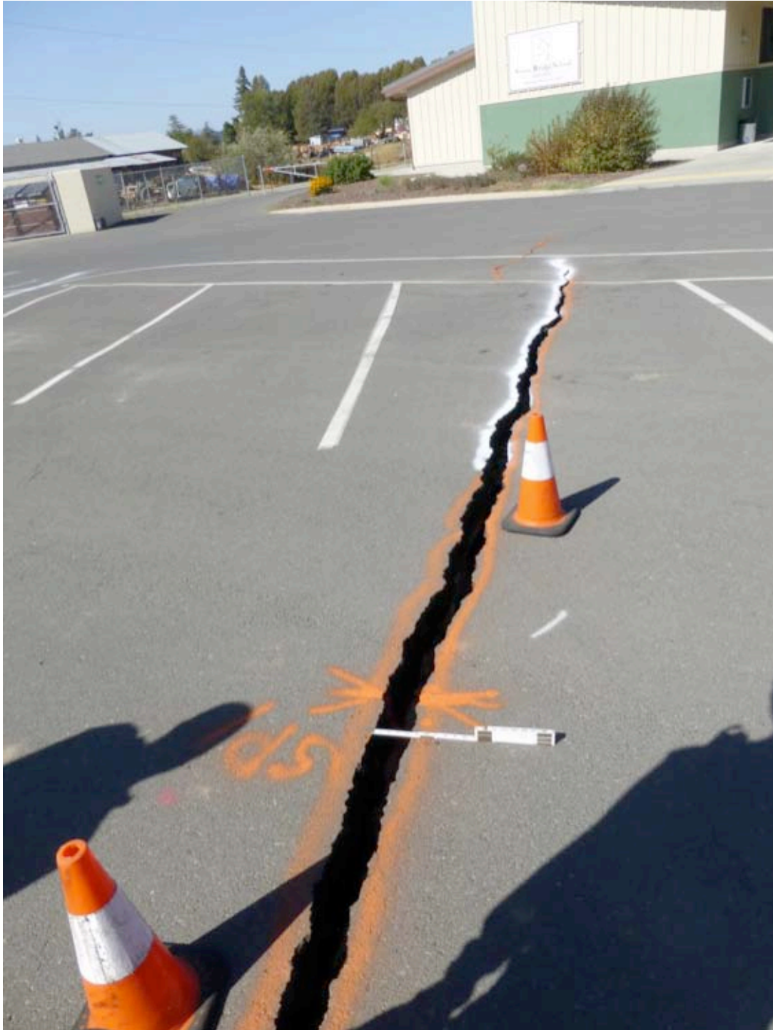
Figure 2-28. Parking lot crack, looking northerly
