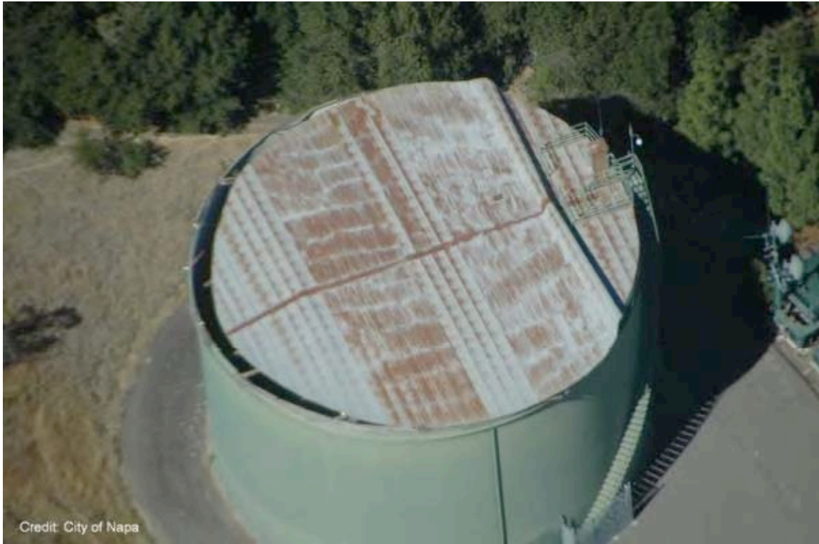
Figure 4-8. Damaged Roof of Steel Tank "B"
