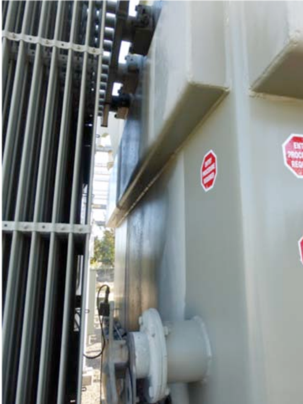
Figure 3-4. Transformer Oil Leak
