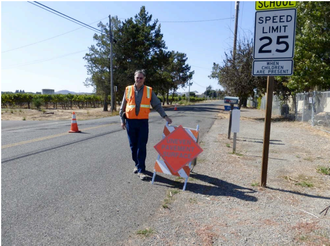
Figure 2-24. Repaired cracks in street
