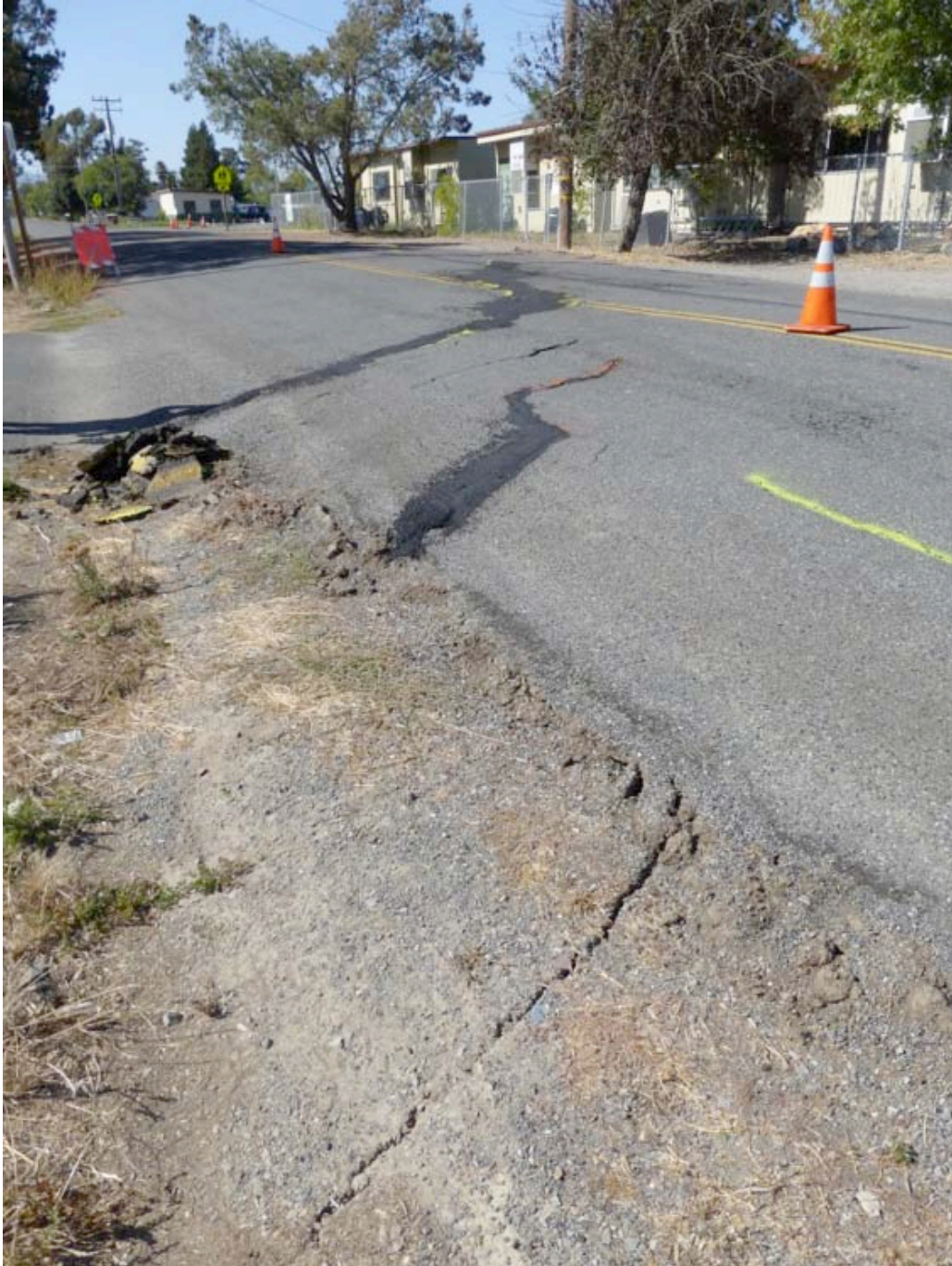
Figure 2-26. Road cracks (repaired and new), looking northerly
