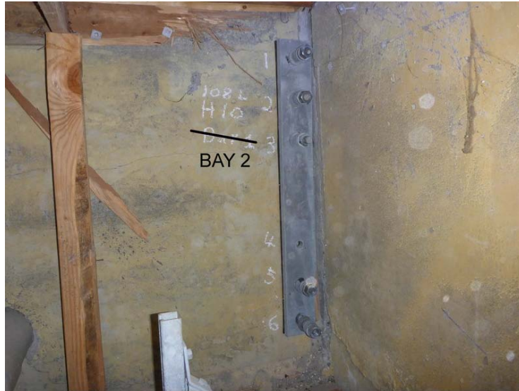
Figure 5-18. Restrainer damage at Hinge 10, Bay 2 of Napa River (W. Imola Ave) Bridge
