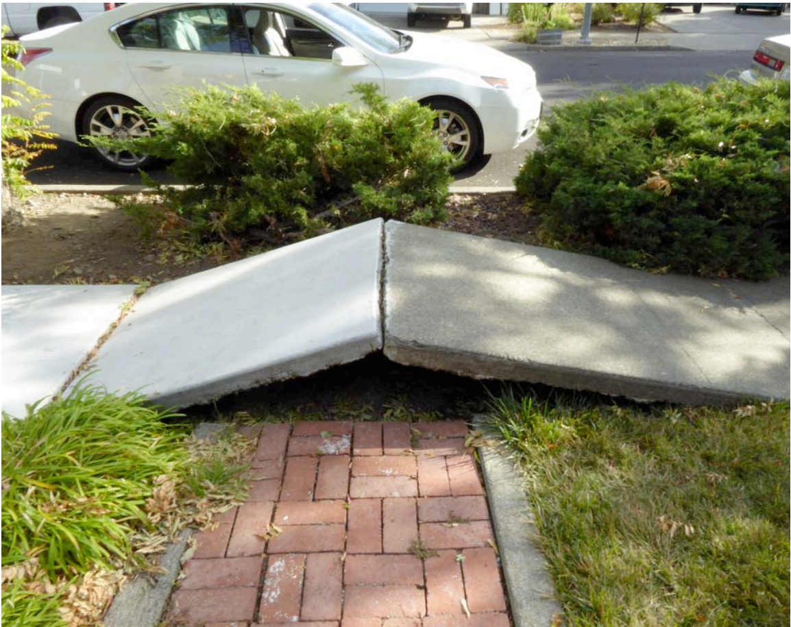
Figure 2-21. Buckled Sidewalk at Fault Offset Location
