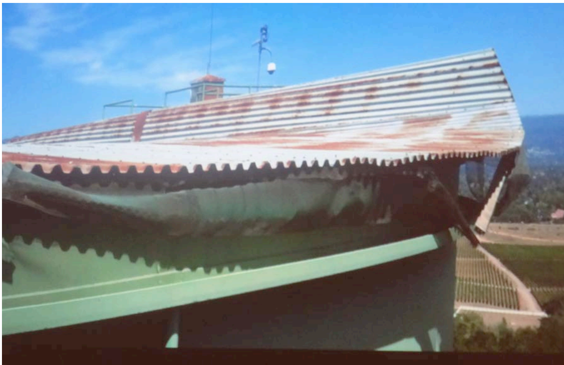
Figure 4-9. Damaged Roof of Steel Tank "B"
