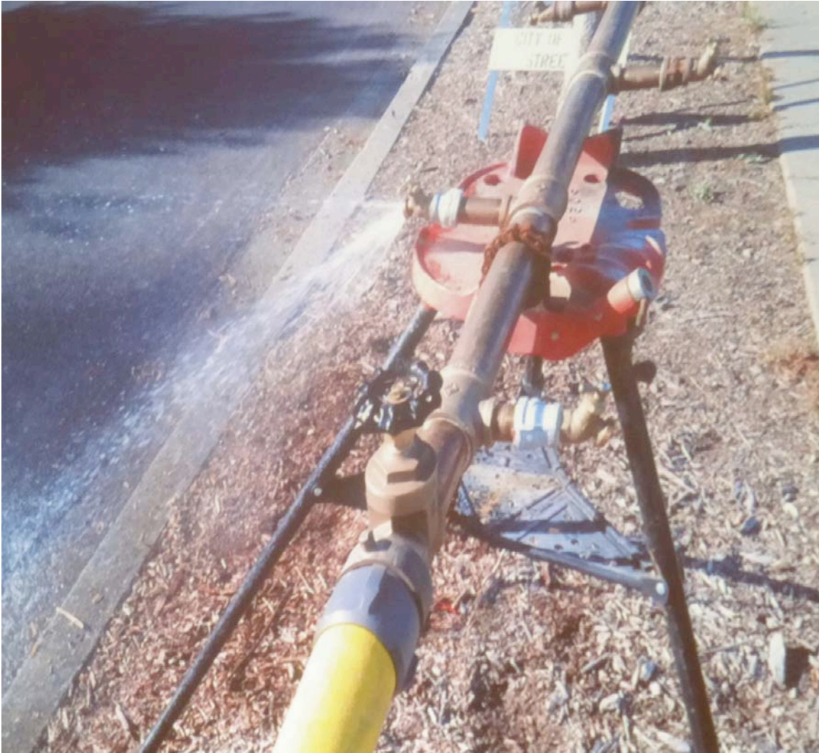
Figure 4-15. Hose Bib Used During Recovery
