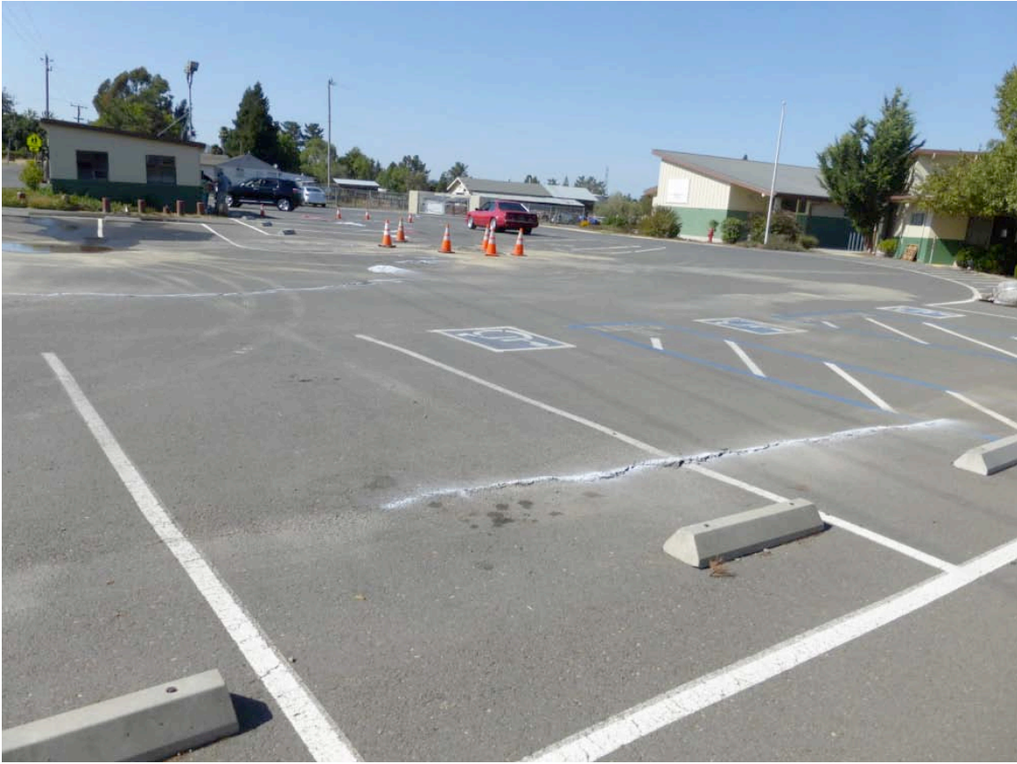
Figure 2-27. Parking lot cracks, looking northerly
