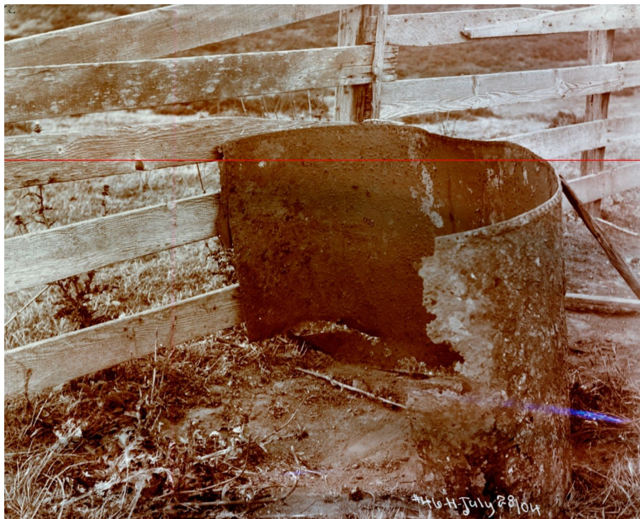
Figure 3. Failure of Pilarcitos 30-inch Low Pressure Pipe (WI-Thin), July 28 1904
