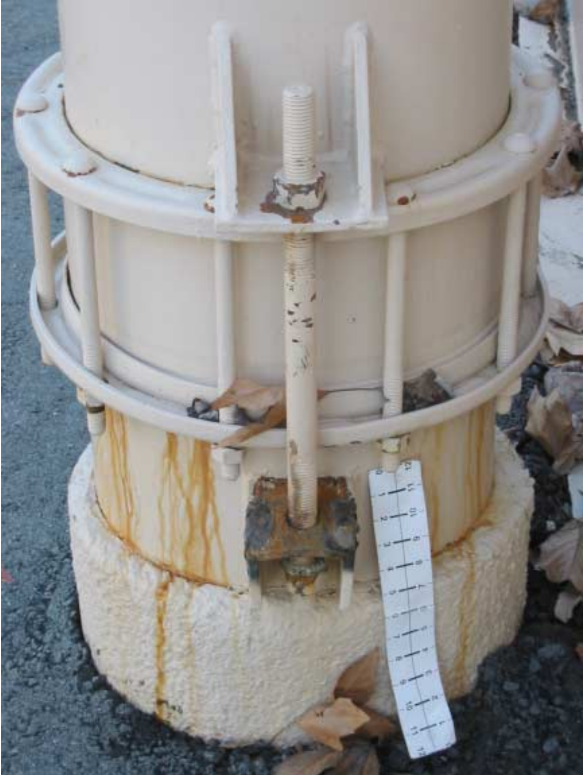
Figure 2. North Tank, Inlet Pipe with Pulled Apart Coupling
