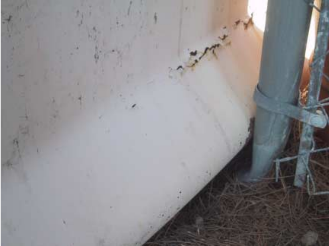
Figure 9. Buckle and Impacted Fence Post
