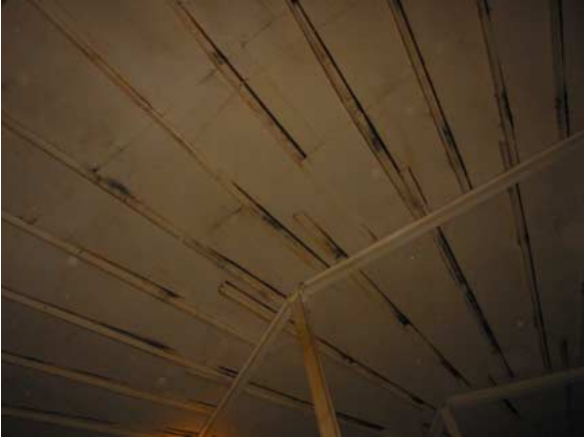
Figure 5. North Tank, Displaced Roof Rafters
