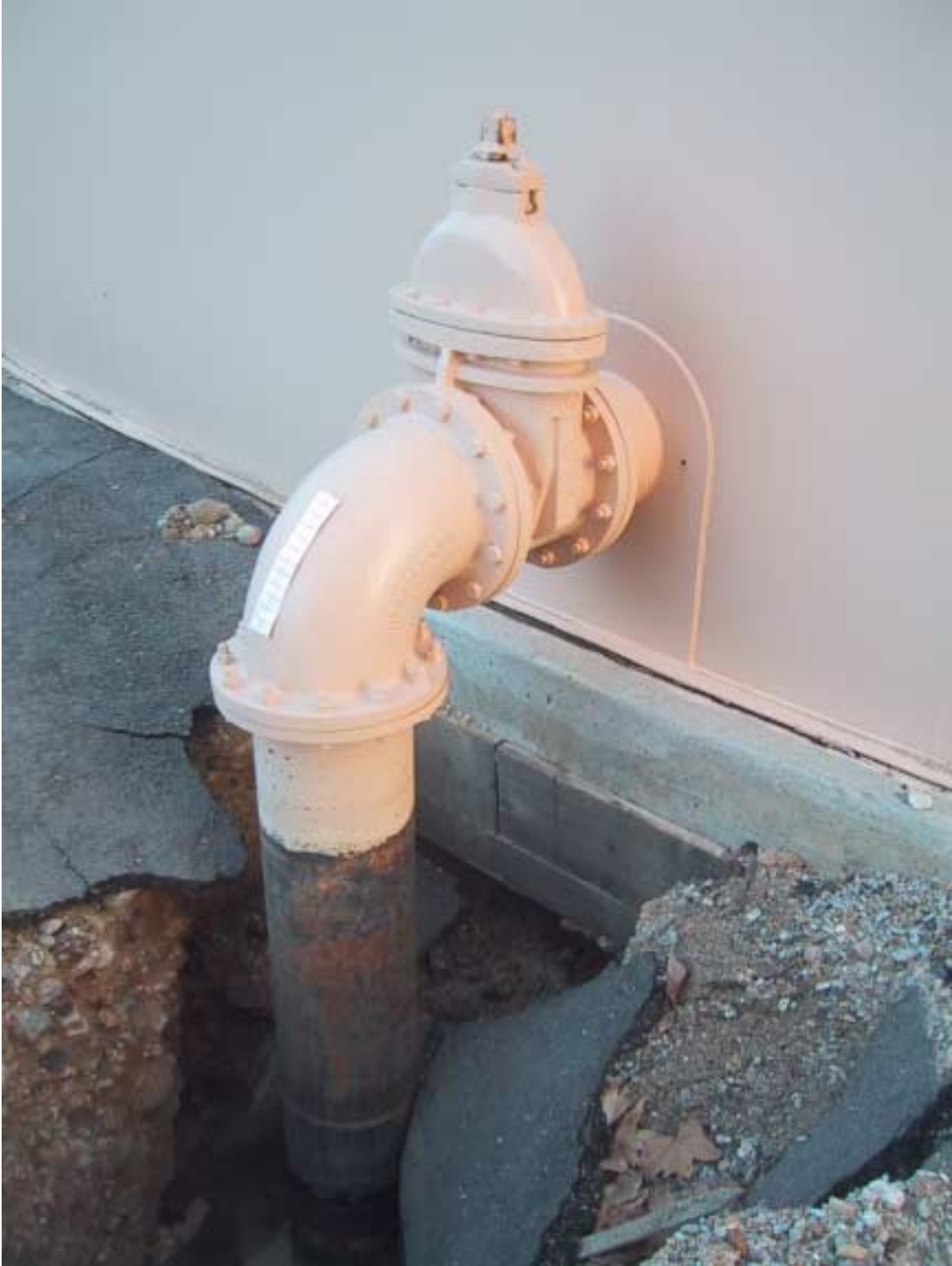
Figure 7. South Tank, Uplift Failed this Side Entry Pipe (pull apart joint under the ground)
