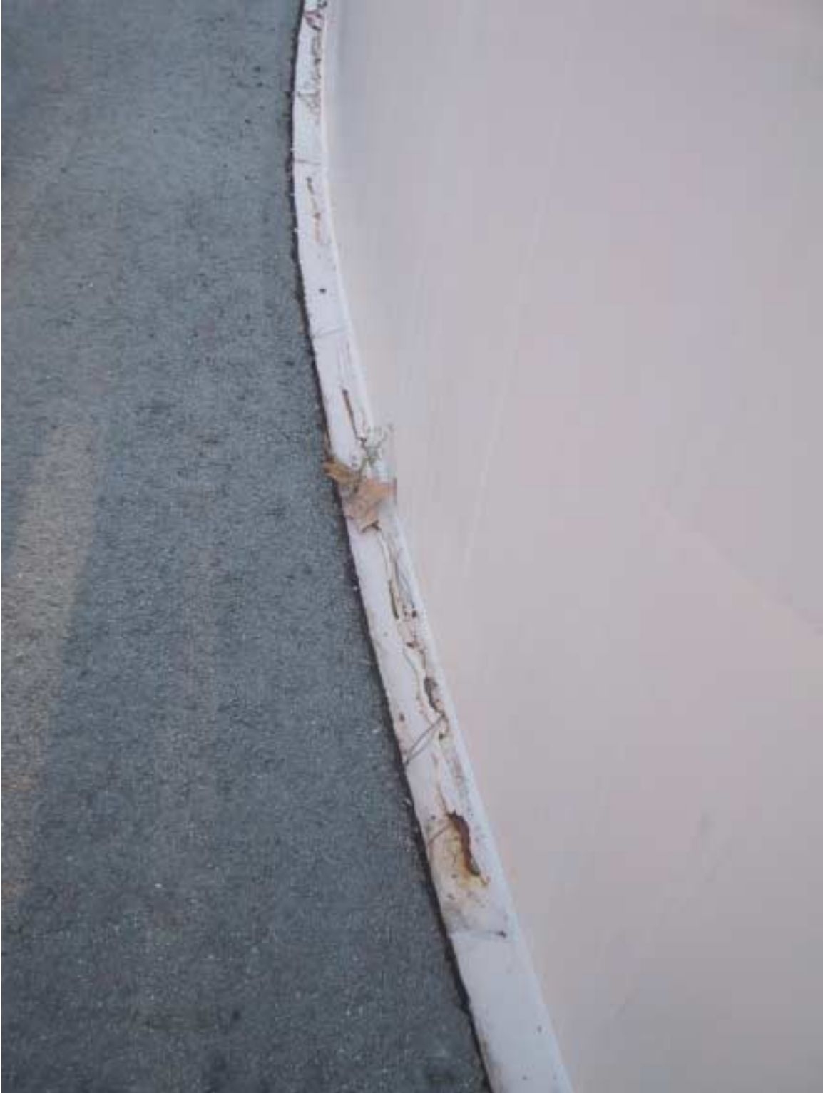
Figure 3. North Tank, Cracking of Paint on Bottom Base Plate
