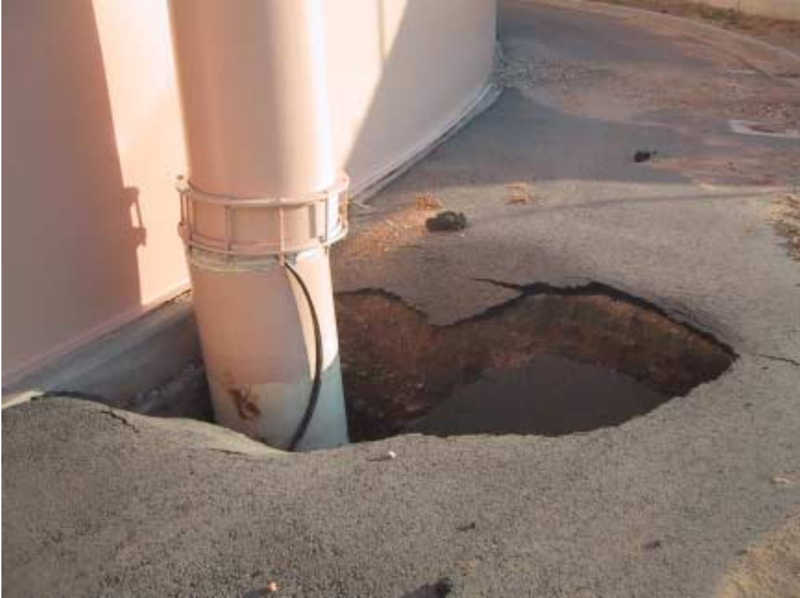
Figure 6. South Tank, Inlet Part Pulled Apart
