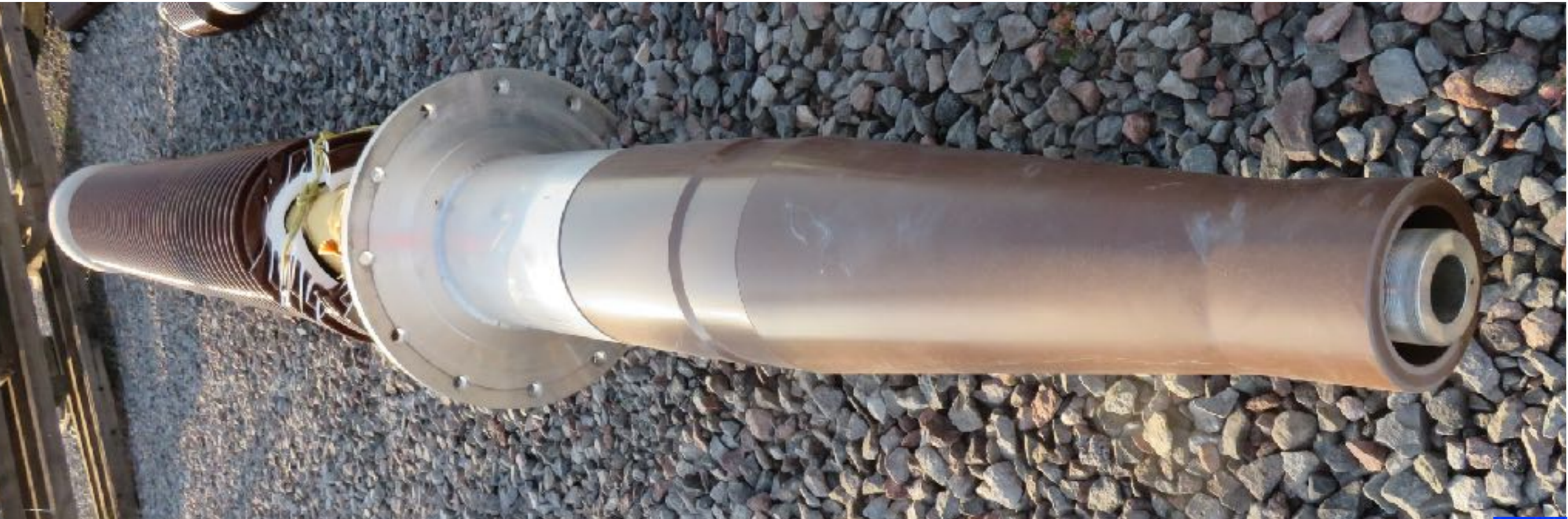
400 kV TR Bushing
