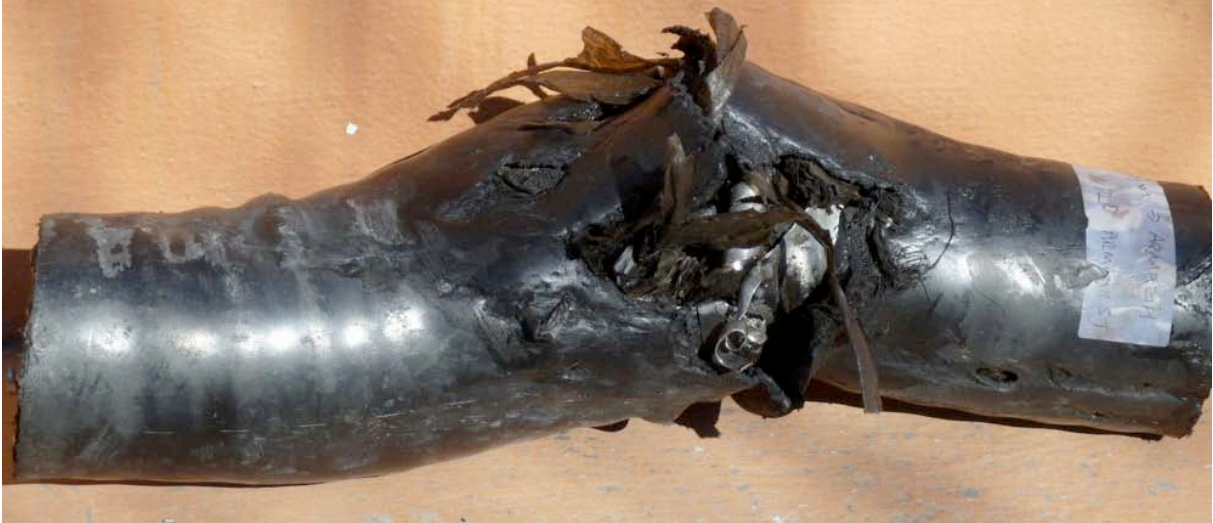
Figure 7. Oil-Type Cable (Location 3)
