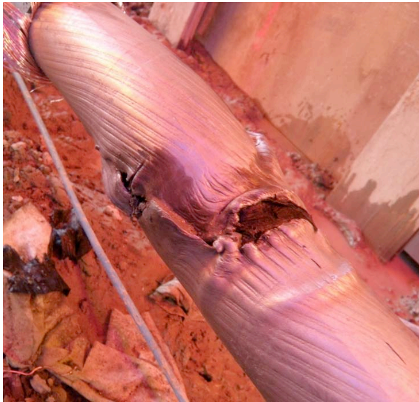
Figure 12. Failed XLPE-Type Cable, Location 4
