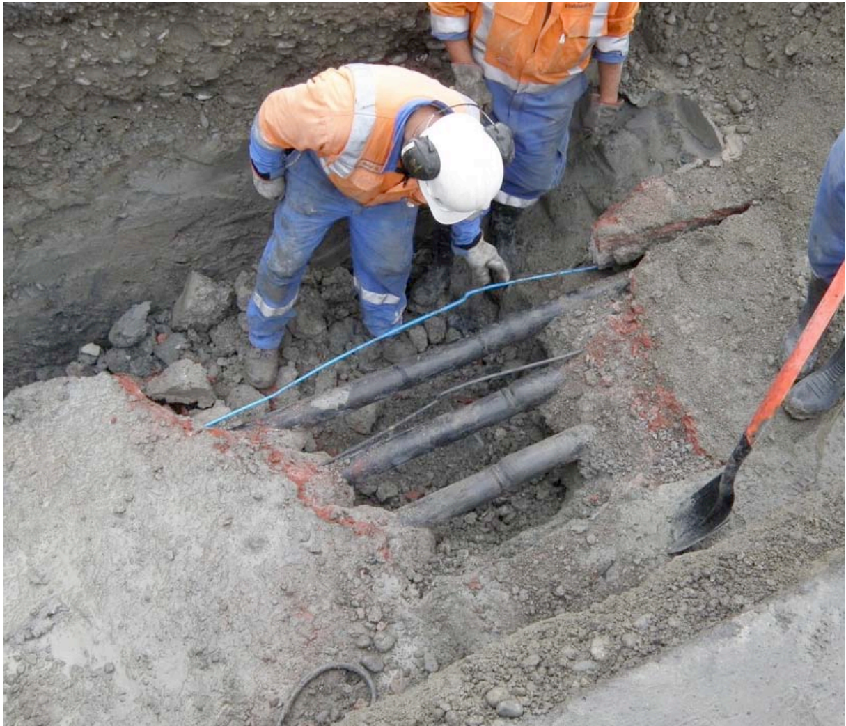
Figure 10. Exposing the Damaged XLPE-Type Cables, Location 6
