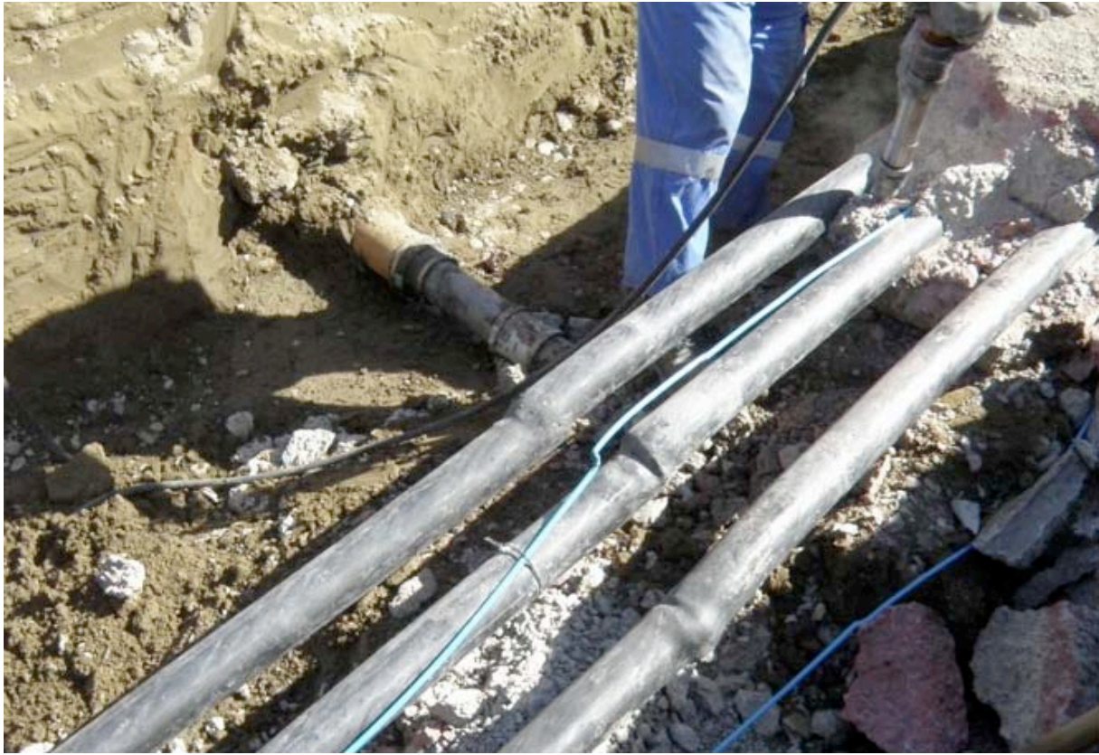
Figure 13. Failed XLPE-Type Cable, Location 5
