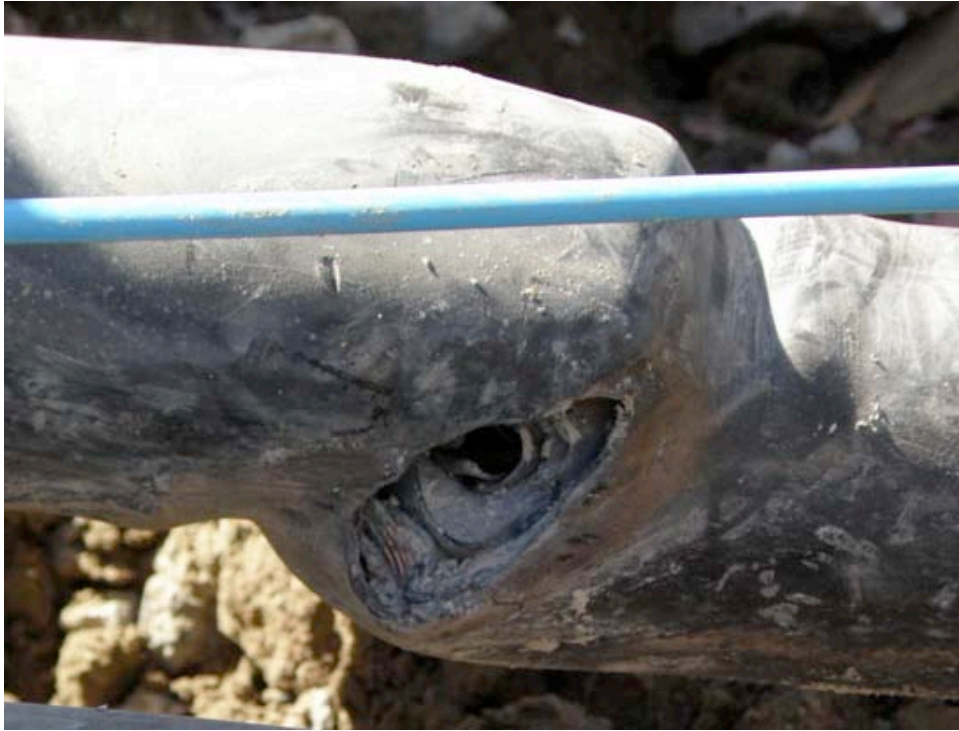
Figure 11. Failed XLPE-Type Cable, Location 4
